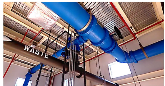
Figure 1 - Franklin WTP Valve Access Area
