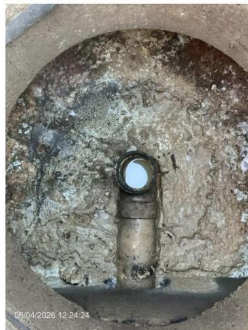
Grease Control Equipment 06/04/2026 Outlet tee
