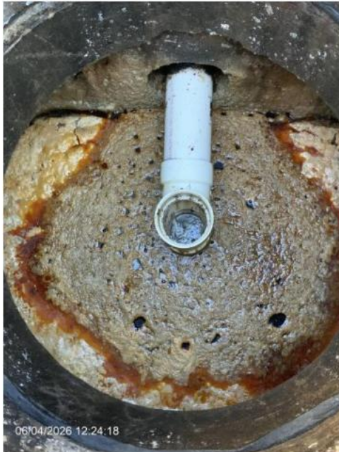
Grease Control Equipment 06/04/2026 Inlet tee
