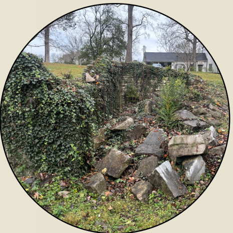
SPRINGHOUSE (COLLAPSED) 1902 - CONTRIBUTING
