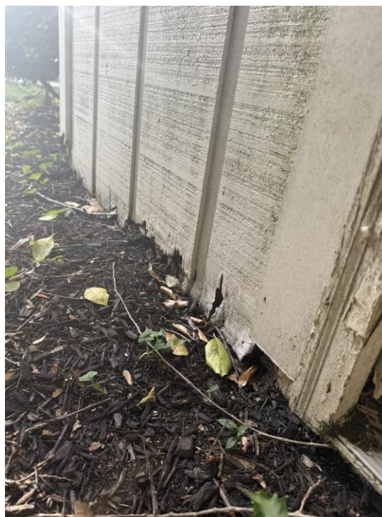
Photo 6 — Corner post base: complete void where wood material has disintegrated
