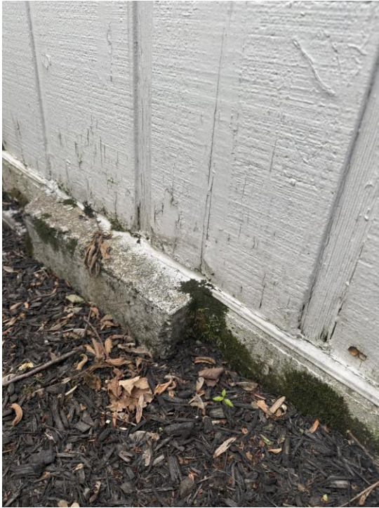
Photo 3 — Base course with moss growth and complete paint failure along foundation line
