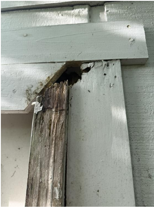
Photo 7 — Close-up of exposed corner post interior: fibrous, split wood with zero sound material
