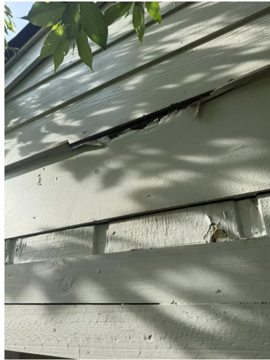
Photo 8 — Mid-wall siding separation with open gap to sheathing layer
