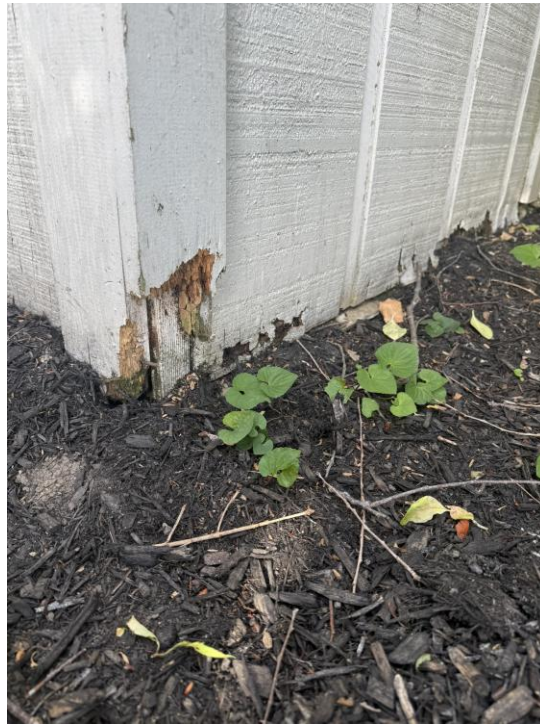
Photo 9 — Additional corner post rot: complete failure of base trim and corner board
