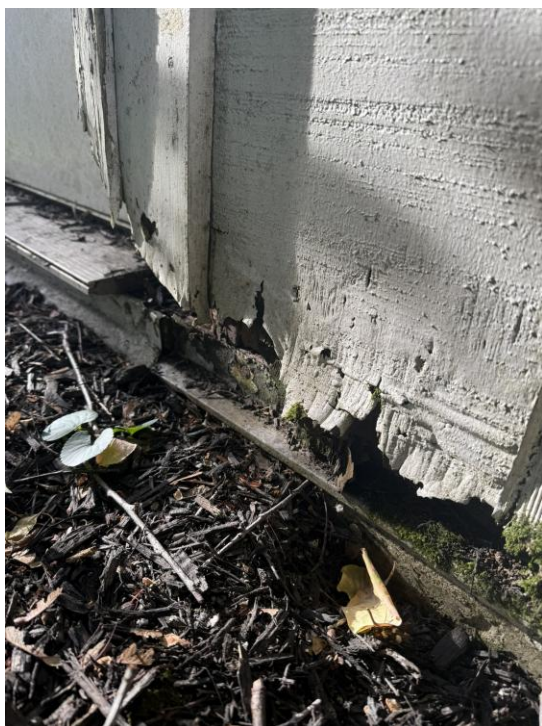
Photo 5 — Corner post with outer casing separated; rotted structural core exposed
