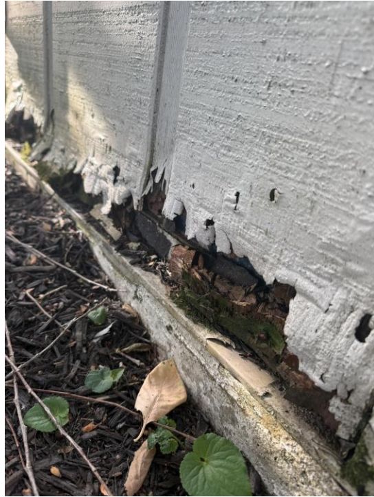
Photo 4 — Advanced rot at base siding: material has crumbled away, leaving open voids
