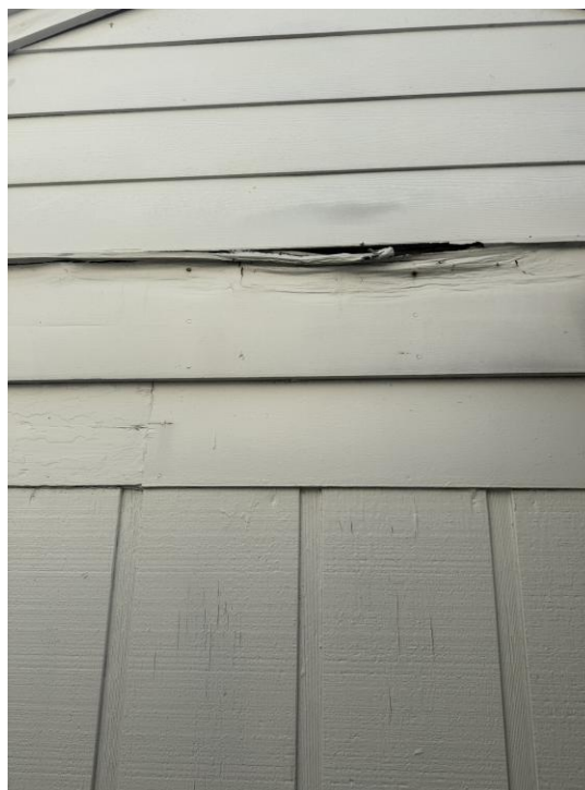
Photo 2 — Second location: siding separation with open void; deterioration migrating into structurally intact neighboring material
