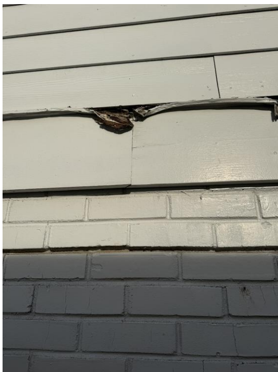
Photo 1 — Buckled siding board split open; rotted substrate exposed and decay visibly spreading into adjacent sound structure
