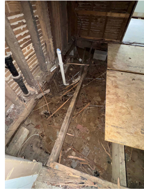
D. HISTORIC JOISTS HAVE COLLAPSED INTO CRAWL SPACE DUE TO TERMITE DAMAGE.
