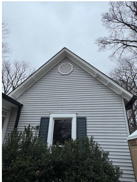
E. FRONT GABLE SHOWS THREE RAFTER TAILS ON EACH SIDE OF THE GABLE WITH NONE AT THE PEAK. THIS IS INDICATIVE OF A DECORATIVE ELEMENT THAT HAS BEEN REMOVED.
