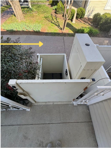
The arrow indicates the driveway. The lift is about 10 feet from the sidewalk at the side of the house.
