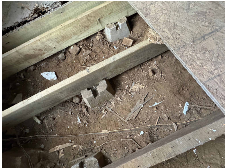
D. CMU SUPPORTS UNDER "NEW" FRAMING. BEARING ON DIRT.
