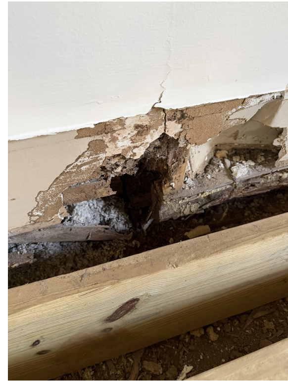
G. PERIMETER SILL BEAM COMPLETELY DETERIORATED.
