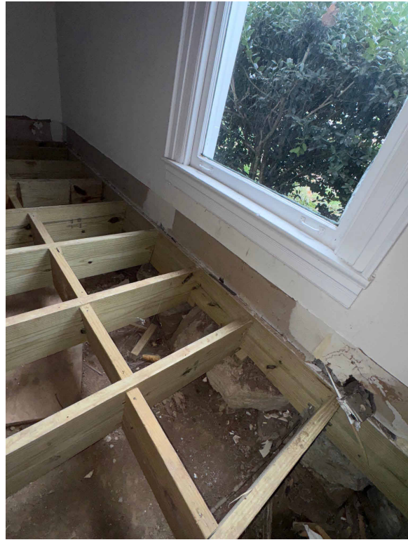
A. RUBBLE FOUNDATION UNDER FRONT GABLE. BEARING ON DIRT.
