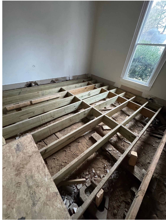
A. NEW FRAMING AT LOCATIONS THROUGHOUT. JOISTS ARE NOT LEVEL AND THERE IS DEFLECTION AMONG JOIST. NO HANGERS OR PROPER FASTENERS.
