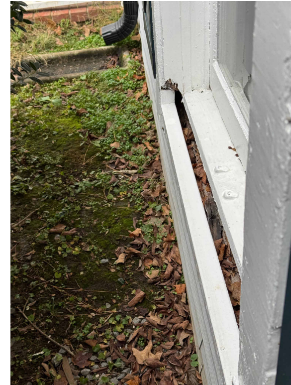
D. THE SILL IS MISSING FROM THE FRONT WINDOW. THE WALL STUDS AND FOUNDATION IS VISIBLE THROUGH THIS HOLE.
