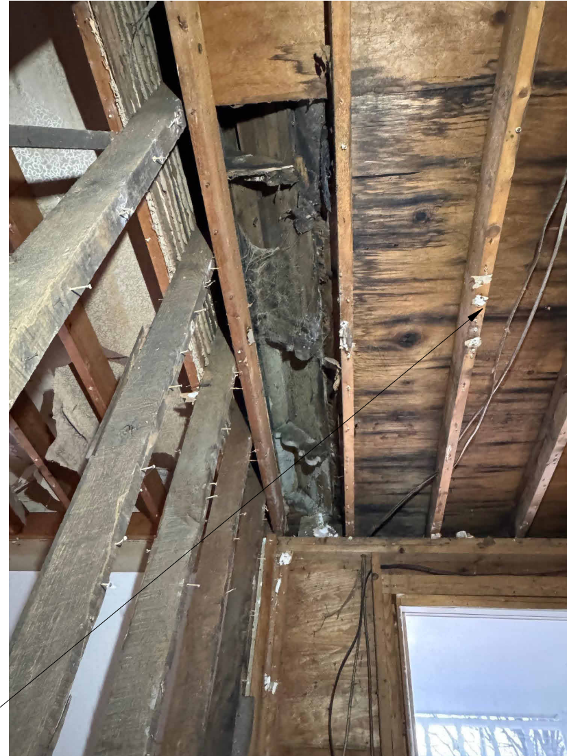
B. EXPOSED RAFTER TAILS FROM FRONT GABLE SEEN INSIDE OF FRONT ROOM CEILING. THIS INDICATES THAT THE PORCH ROOF SLOPE WOULD HAVE BEEN LOWER THAN THESE RAFTER TAILS AND THESE WOULD HAVE BEEN SEEN FROM THE FRONT OF THE HOUSE.
