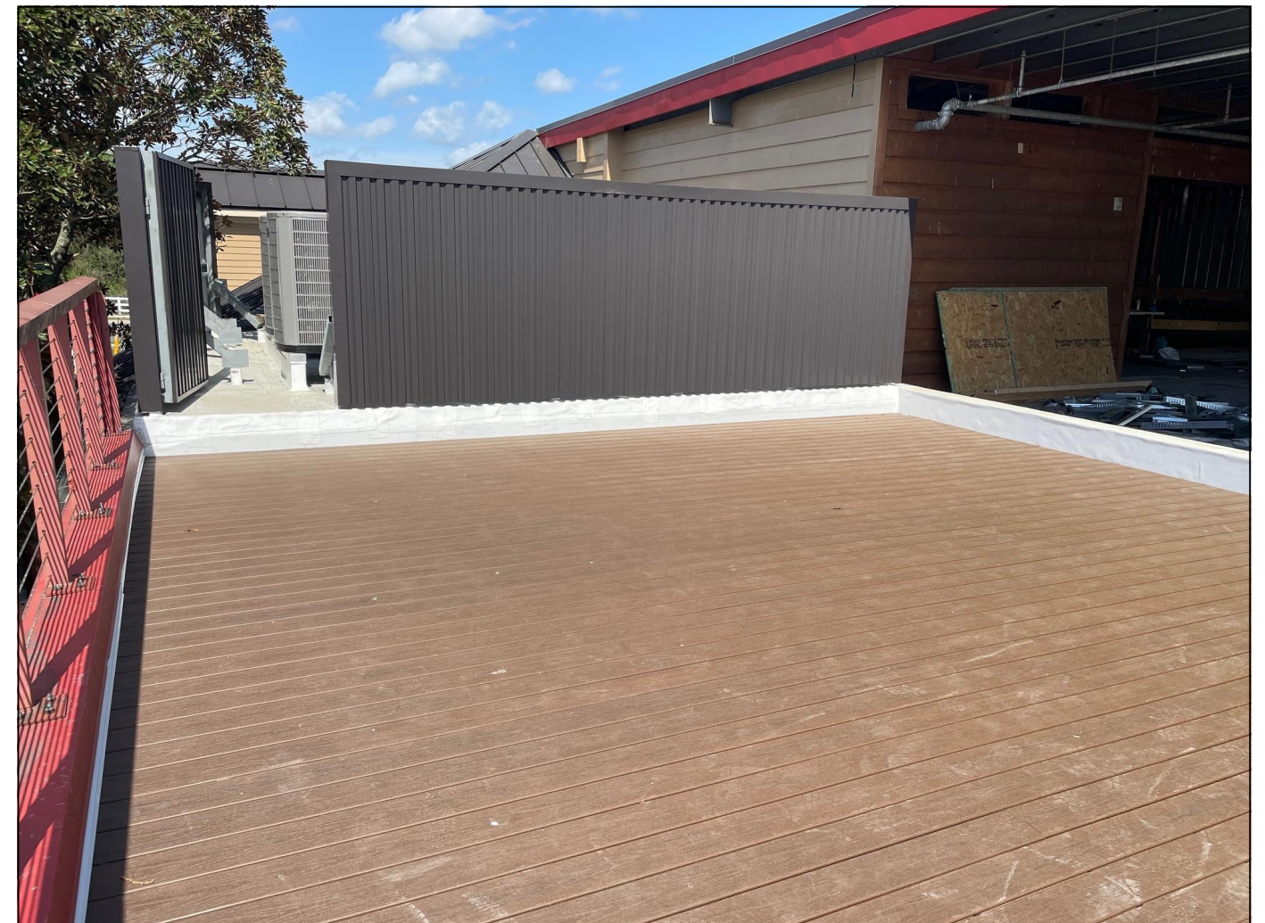
EXISTING: NEWLY INSTALLED METAL SCREENING AS SEEN FROM THE 2nd FLOOR DECK.
