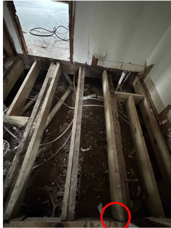
C. NEW FRAMING AT INTERIOR LOCATIONS. SISTERD ALONG JOISTS WITH GAPS AND NO FASTENERS.
