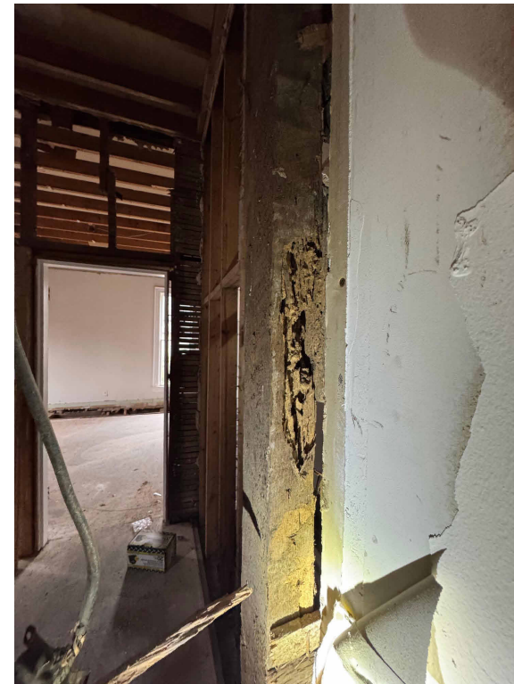
G. TERMITE DAMAGE AT APPROX 5' ABOVE FLOOR
