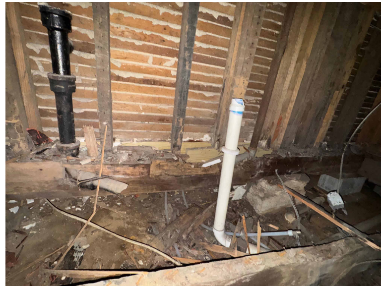
F. TERMITE DAMAGE IN BOTH THE FLOOR JOISTS AND VERTICAL FRAMING
