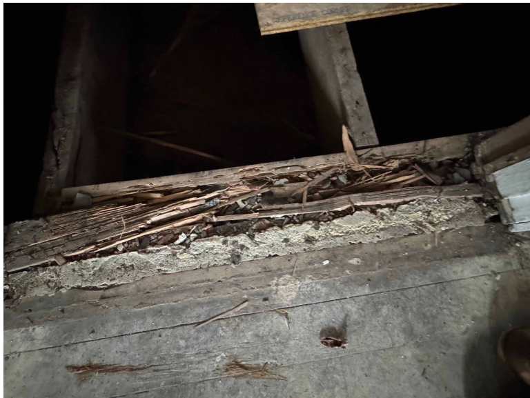
E. CLOSE UP OF TERMITE DAMAGE
