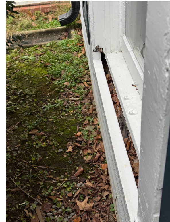
D. THE SILL IS MISSING FROM THE FRONT WINDOW. THE WALL STUDS AND FOUNDATION IS VISIBLE THROUGH THIS HOLE.
