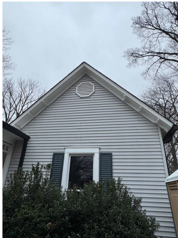
E. FRONT GABLE SHOWS THREE RAFTER TAILS ON EACH SIDE OF THE GABLE WITH NONE AT THE PEAK. THIS IS INDICATIVE OF A DECORATIVE ELEMENT THAT HAS BEEN REMOVED.
