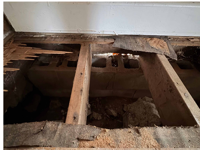
E. DAYLIGHT CAN BE SEEN AT MANY LOCATIONS.
