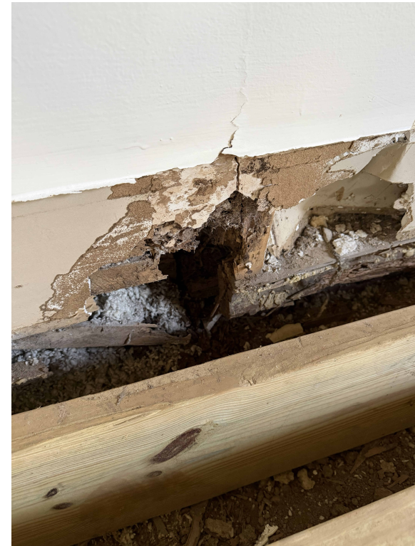
G. PERIMETER SILL BEAM COMPLETELY DETERIORATED.
