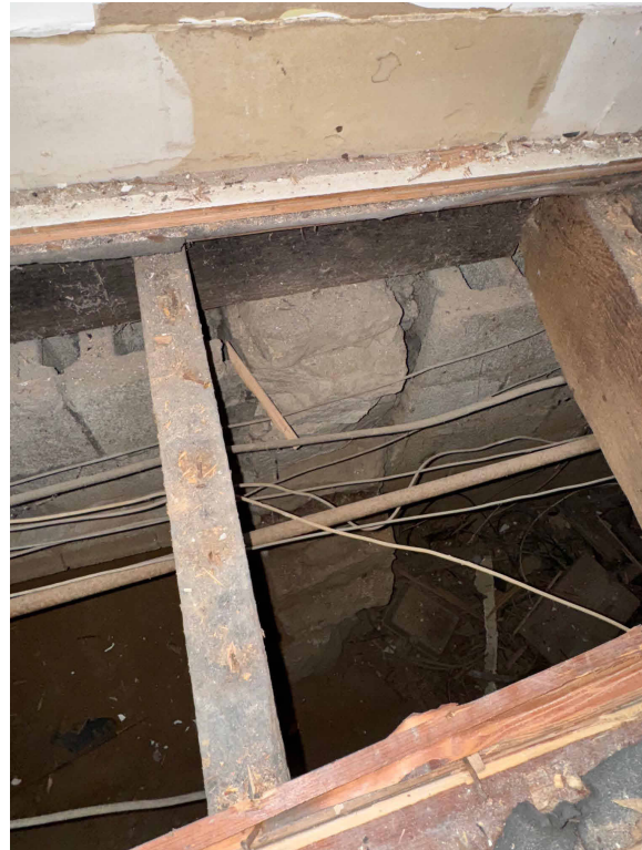
B. MIX OF STONE AND CMU, NOT GROUTED. BEARING ON DIRT
