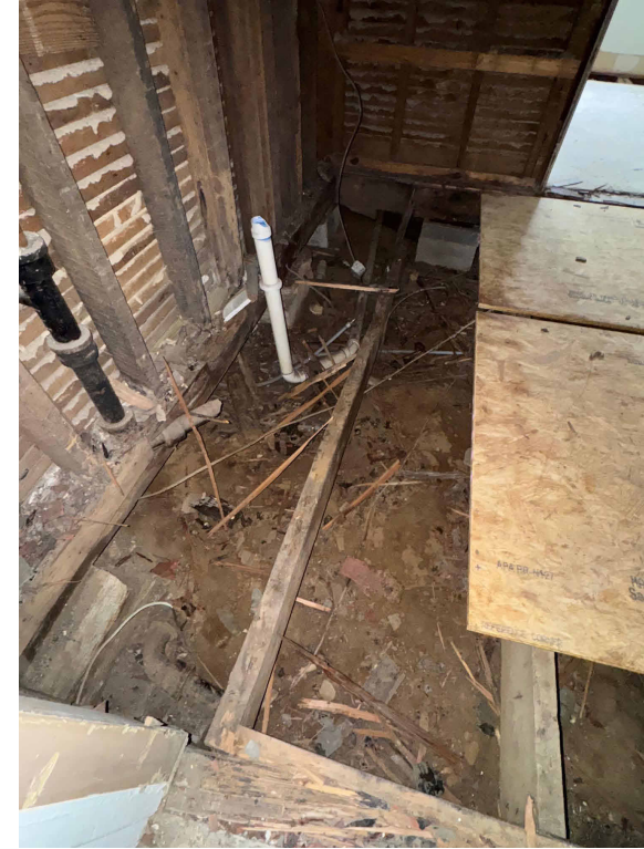
D. HISTORIC JOISTS HAVE COLLAPSED INTO CRAWL SPACE DUE TO TERMITE DAMAGE.
