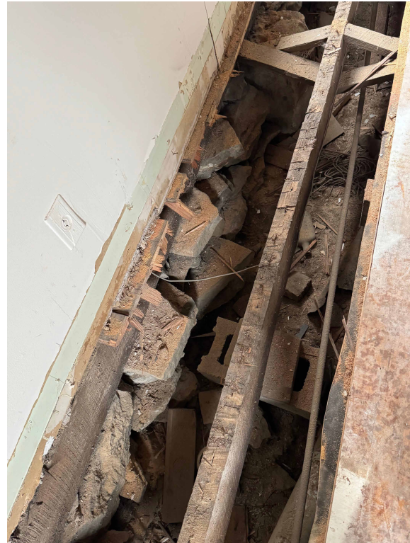
C. RUBBLE FOUNDATION UNDER SIDE GABLE. BEARING ON DIRT.
