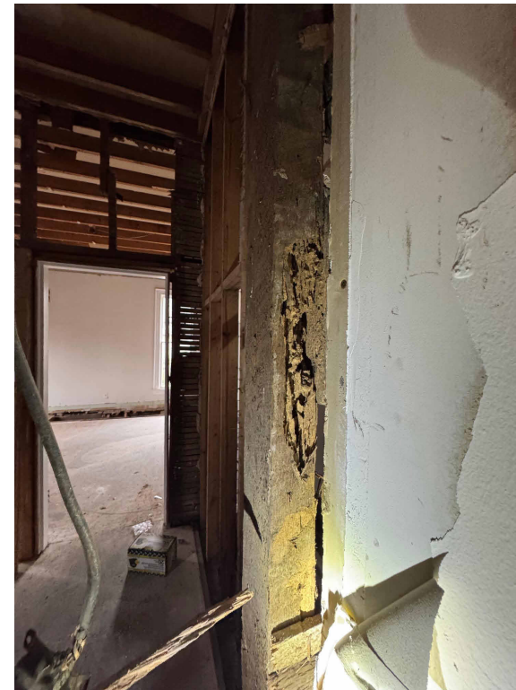
G. TERMITE DAMAGE AT APPROX 5' ABOVE FLOOR
