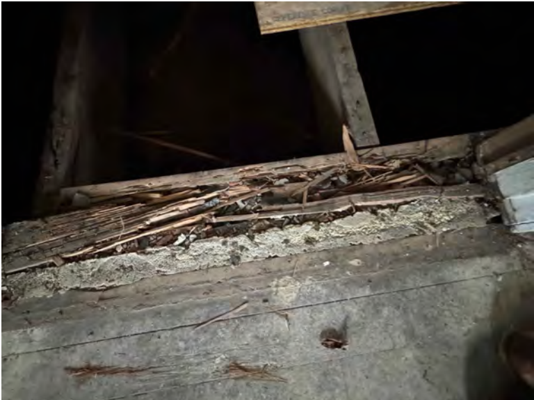
E. CLOSE UP OF TERMITE DAMAGE
