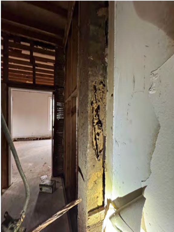
G. TERMITE DAMAGE AT APPROX 5' ABOVE FLOOR
