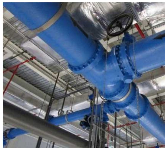
Figure 5 - Franklin WTP Valve Access Area
