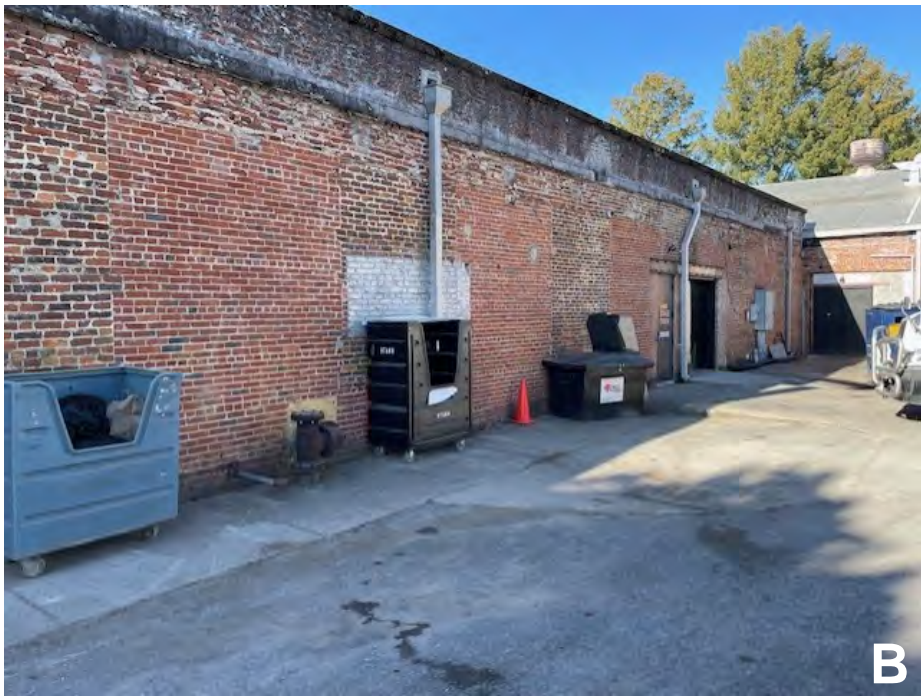
EXISTING BRICK WALLS AT BUILDING 3 ARE NOT REQUIRED TO BE RATED. EXISTING BRICK WALLS AT BUILDING 5 TO HAVE A 2-HR RATING.
