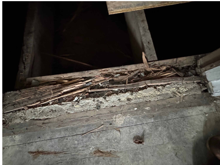
(E) CLOSE UP OF TERMITE DAMAGE
