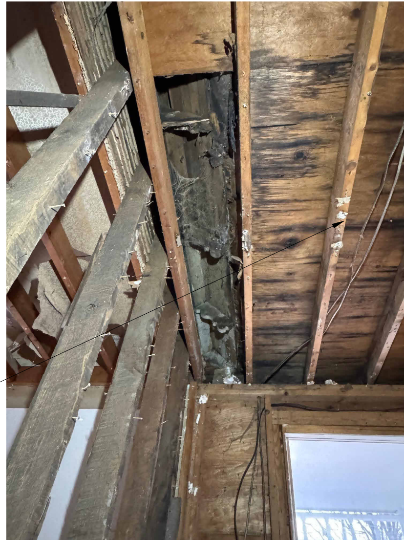
(B) EXPOSED RAFTER TAILS FROM FRONT GABLE VISIBLE ABOVE FRONT ROOM. THIS INDICATES THAT THE PORCH ROOF SLOPE WOULD HAVE BEEN LOWER THAN THESE RAFTER TAILS AND THESE WOULD HAVE BEEN SEEN FROM THE FRONT OF THE HOUSE.
