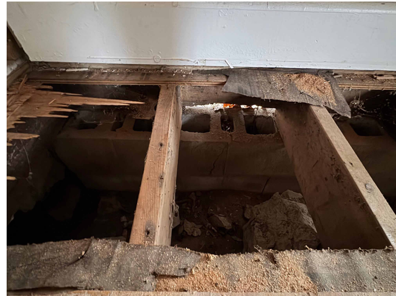
(E) DAYLIGHT CAN BE SEEN AT MANY LOCATIONS BETWEEN WALL AND FOUNDATION.
