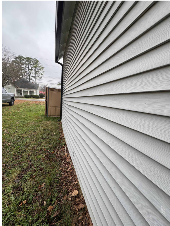
(A) VISIBLE BOW IN EXTERIOR WALL FRAMING
