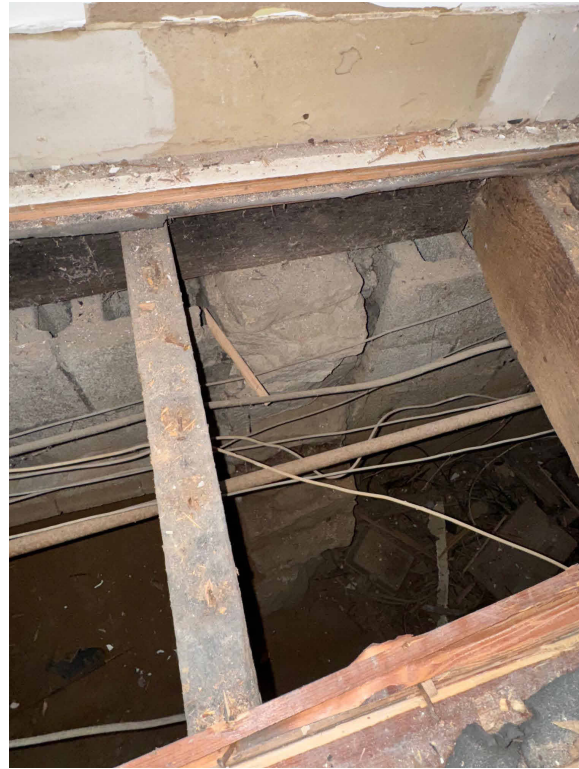
(B) MIX OF STONE AND CMU, NOT GROUDED. BEARING ON DIRT
