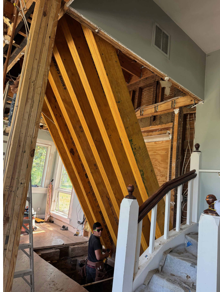
(A) EXAMPLE OF SHORING HOLDING A SECOND FLOOR STRUCTURE WHILE FOUNDATION REPAIRS ARE BEING MADE.
