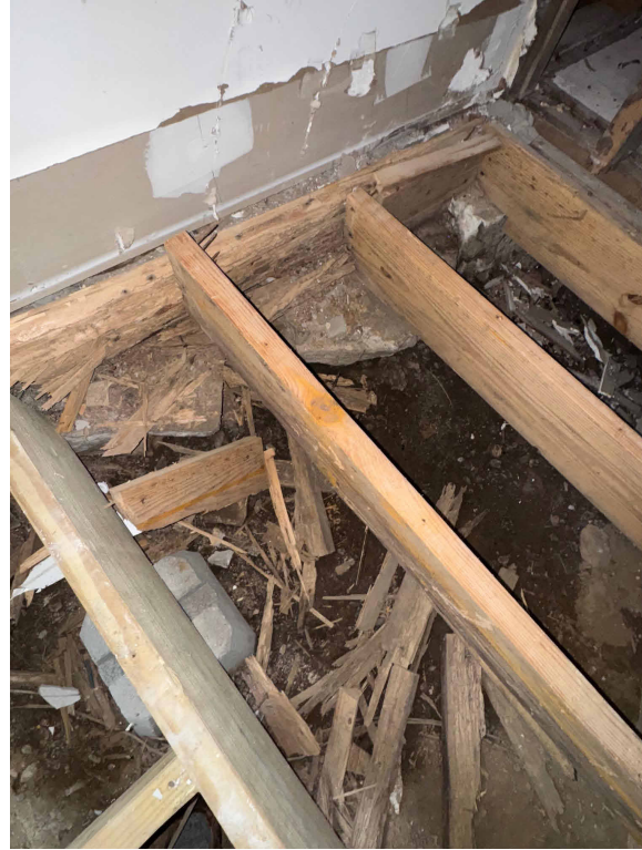
(B) HISTORIC RIM BOARD HAS SEVERE DETERIORATION FROM TERMITE DAMAGE.
