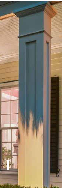
FRONT PORCH COLUMNS - NEW COLUMNS AT REAR SIMILAR TO FRONT PORCH COLUMN STYLE
