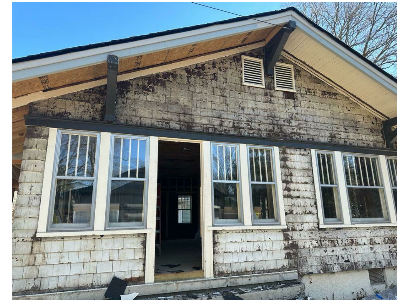
EXISTING SIDING FOUND UNDER ASBESTOS SIDING
