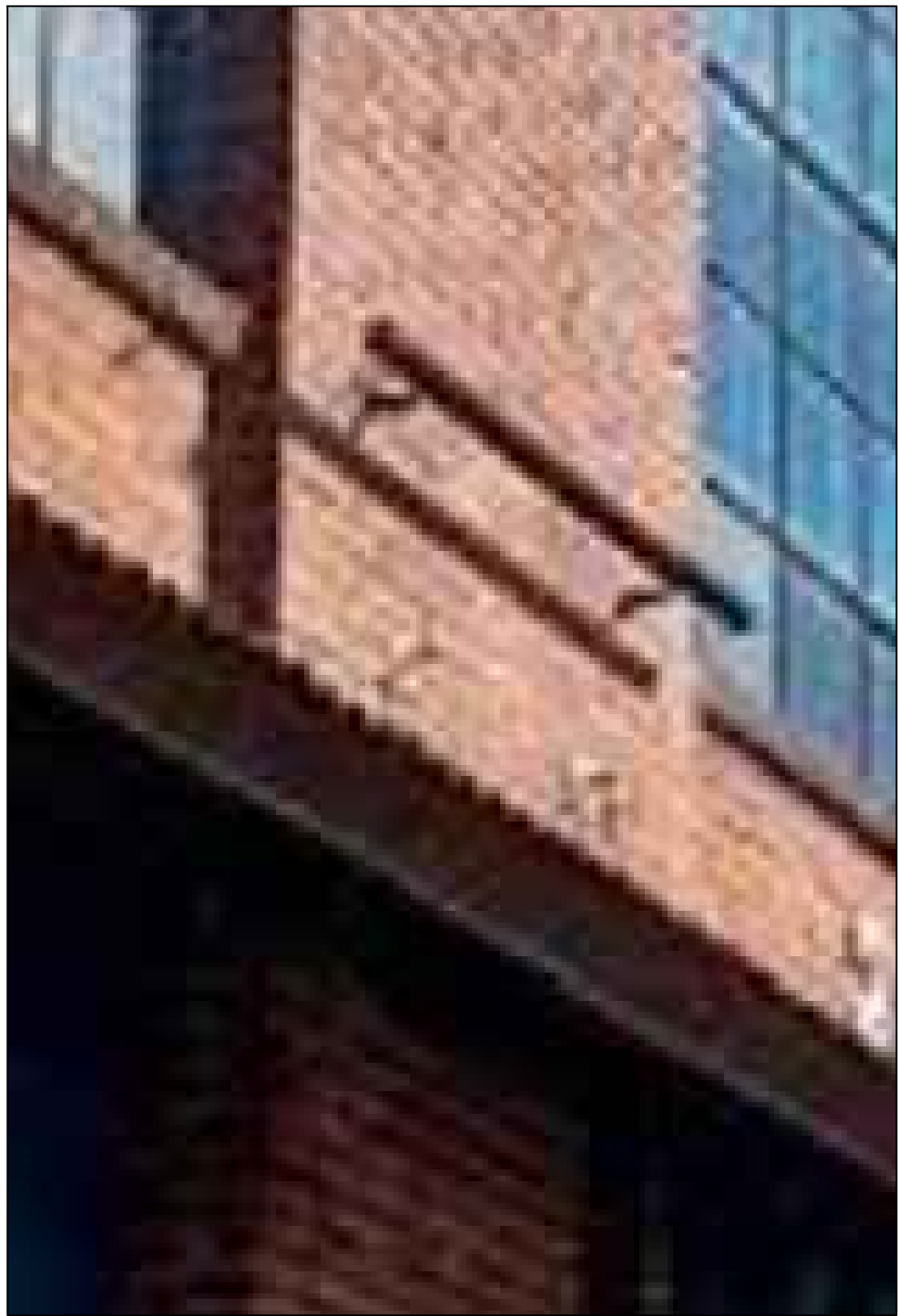
EXISTING LIGHTING ON SITE: SIMPLE LINEAR LIGHTS MOUNTED BACK TO BUILDING TO CAST GLOW ONTO HISTORIC BRICK.
