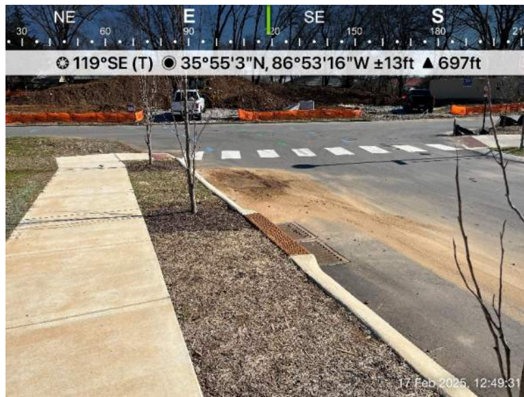
Sediment in Cherokee Roadway entrance, north side of roadway
