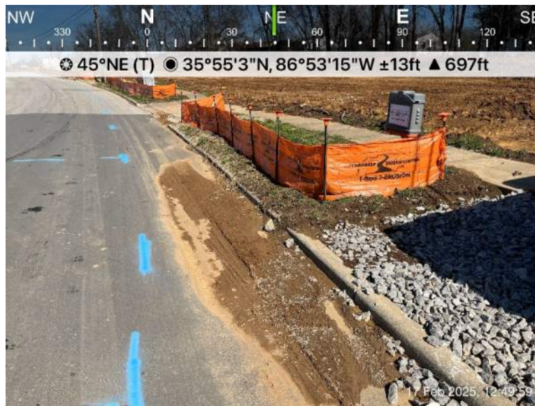
Sediment at curb line on east side of Shawnee Drive at construction entrance
