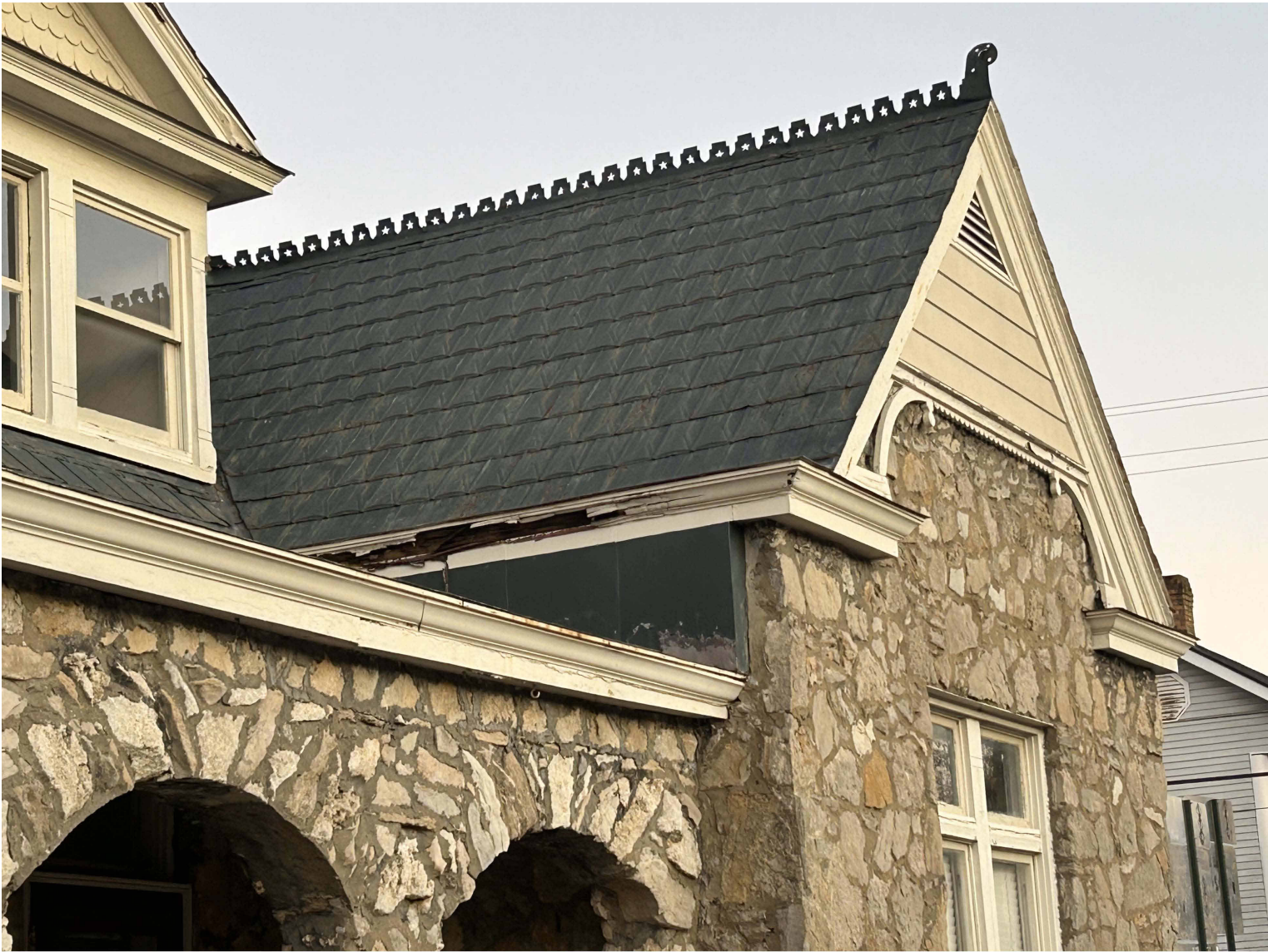
DETERIORATING TRIM ALONG 4TH AVE
