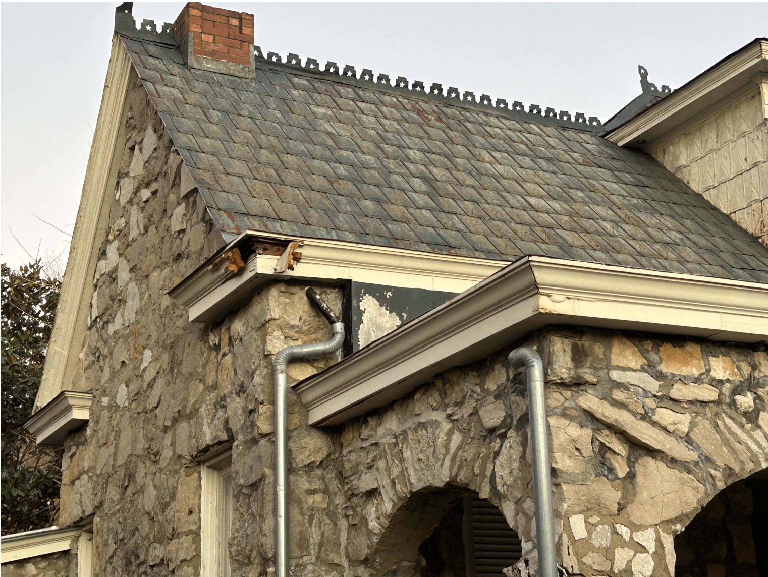
DETERIORATING TRIM ALONG 4TH AVE
