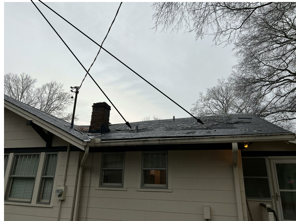
REAR OF HOUSE, SHOWING STRUCTURAL SAG
