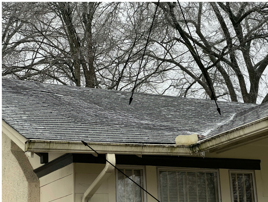
FRONT OF HOUSE, SHOWING STRUCTURAL SAG
