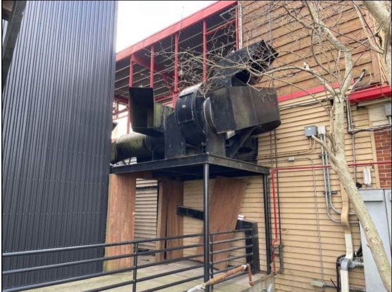
EXISTING HVAC EQUIPMENT TO BE REMOVED
