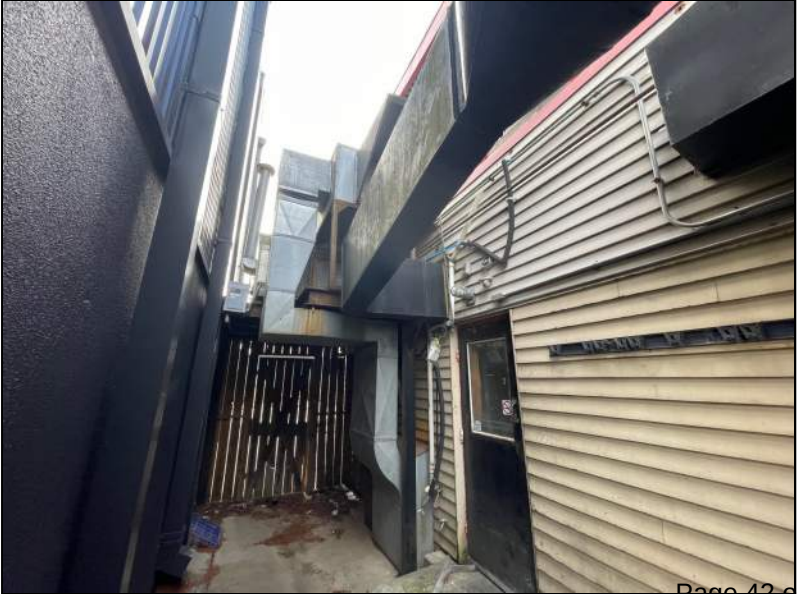
EXISTING HVAC EQUIPMENT TO BE REMOVED
