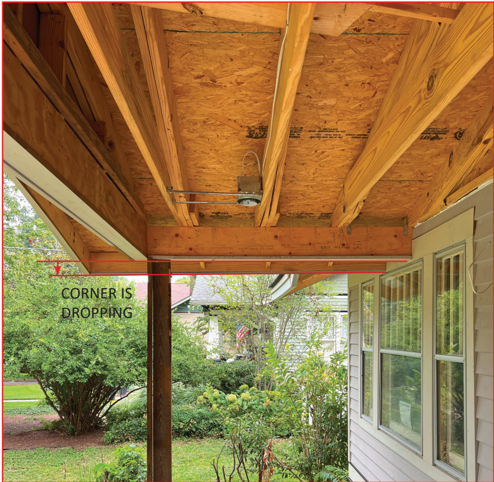
FRONT PROCH ROOF SAGGING
