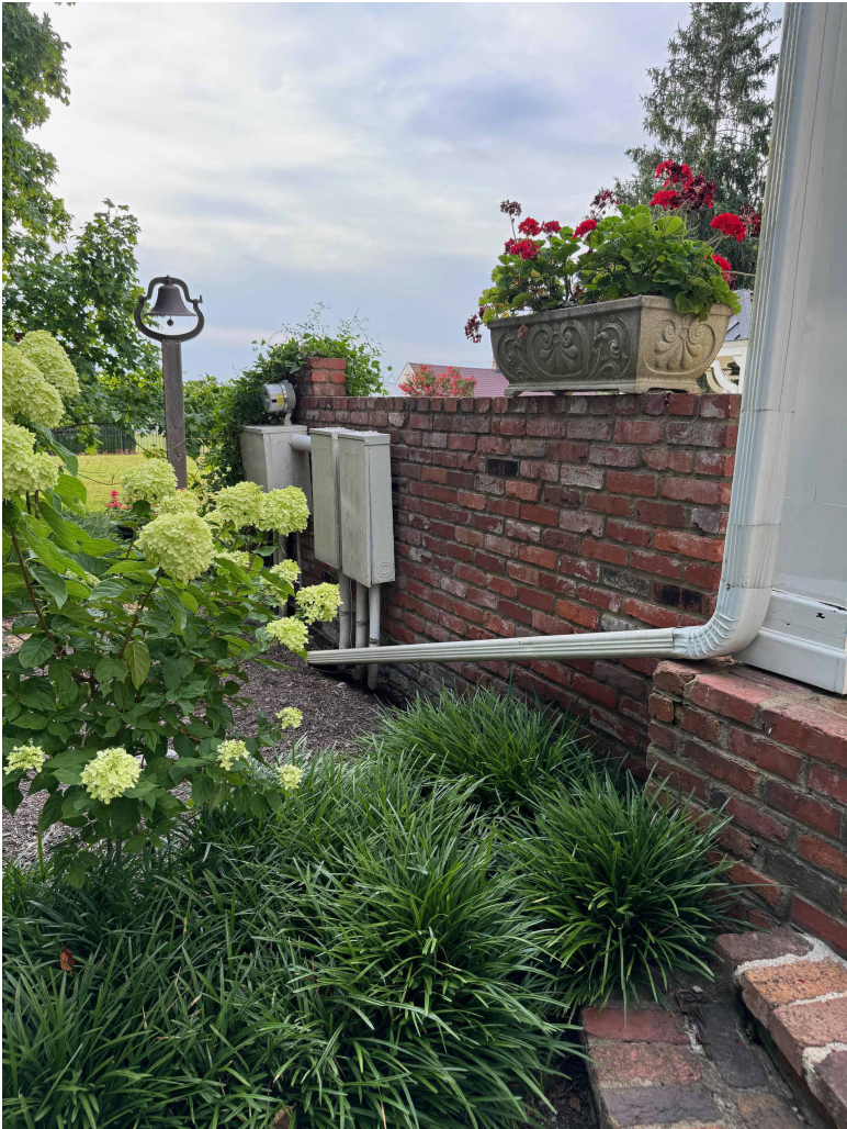
EXISTING ELECTRICAL METERS TO REMAIN
