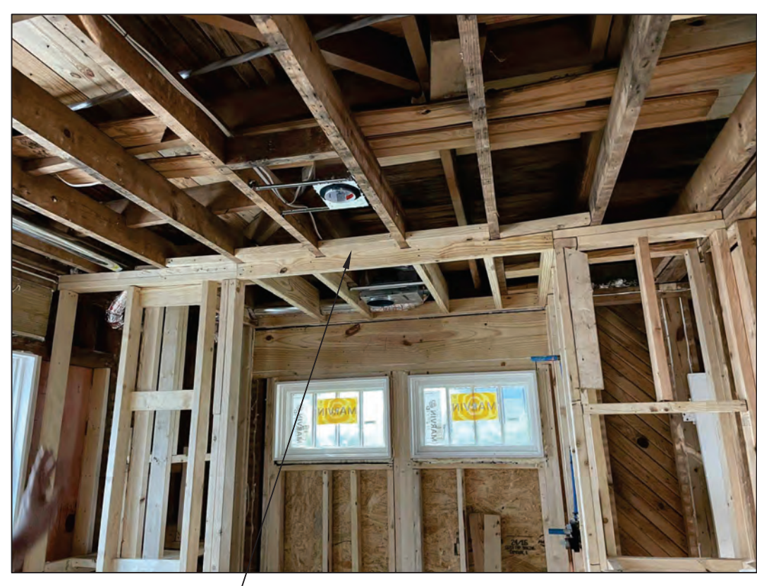
⑥ Inadequate sized header to support new ceiling joists.
