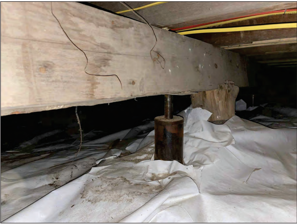
1 Existing Girder exhibits rotation and been supplemented with screw jacks. Straighten beam and support with masonry pier or steel post at 7'-0" max spacing
