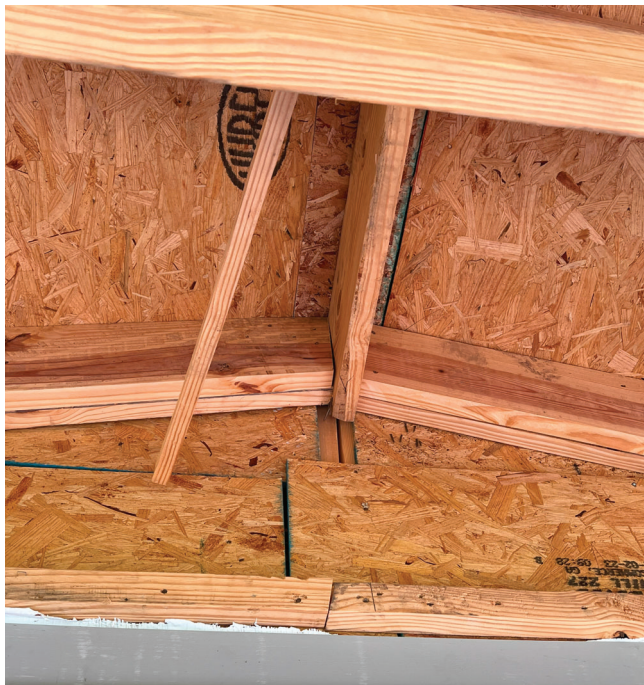
UNSUPPORTED PORCH ROOF CONSTRUCTION
