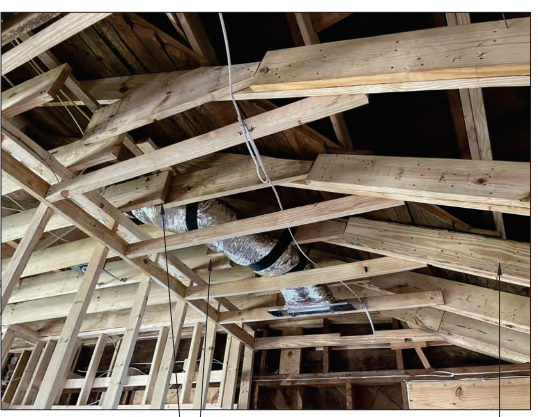
④ Ceiling joist do not align to develop roof thrust. New 2x4 ceiling joist with toe nail connections. Splice rafter extension is inadequate.
