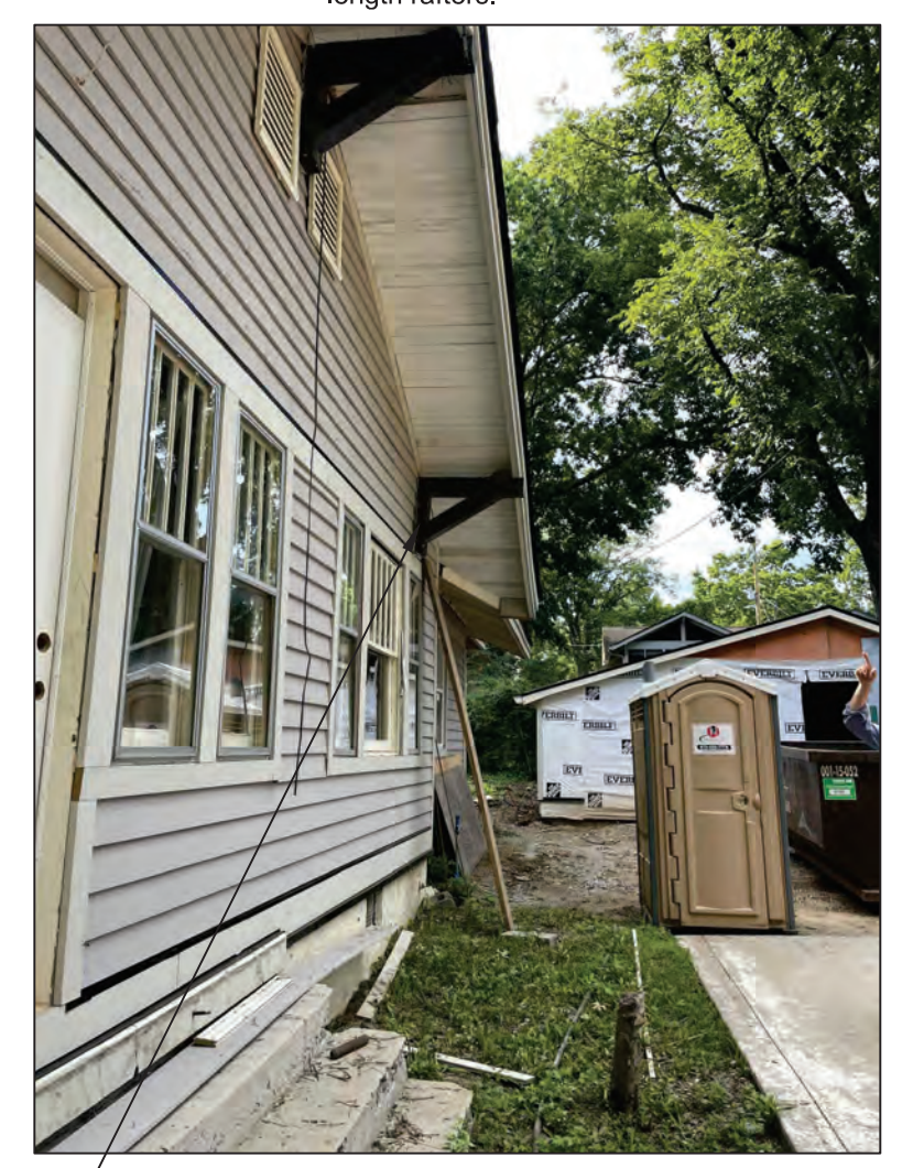
⑨2 No full height studs or bracing back to roof to support exterior bracket. See Photo 9.1
