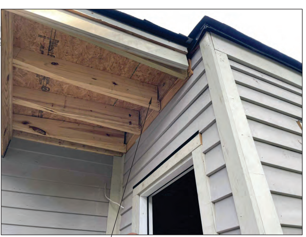
⑦ New porch roof rafters were cut too short and are only toe-nailed in. Replace rafters with correct length rafters.
