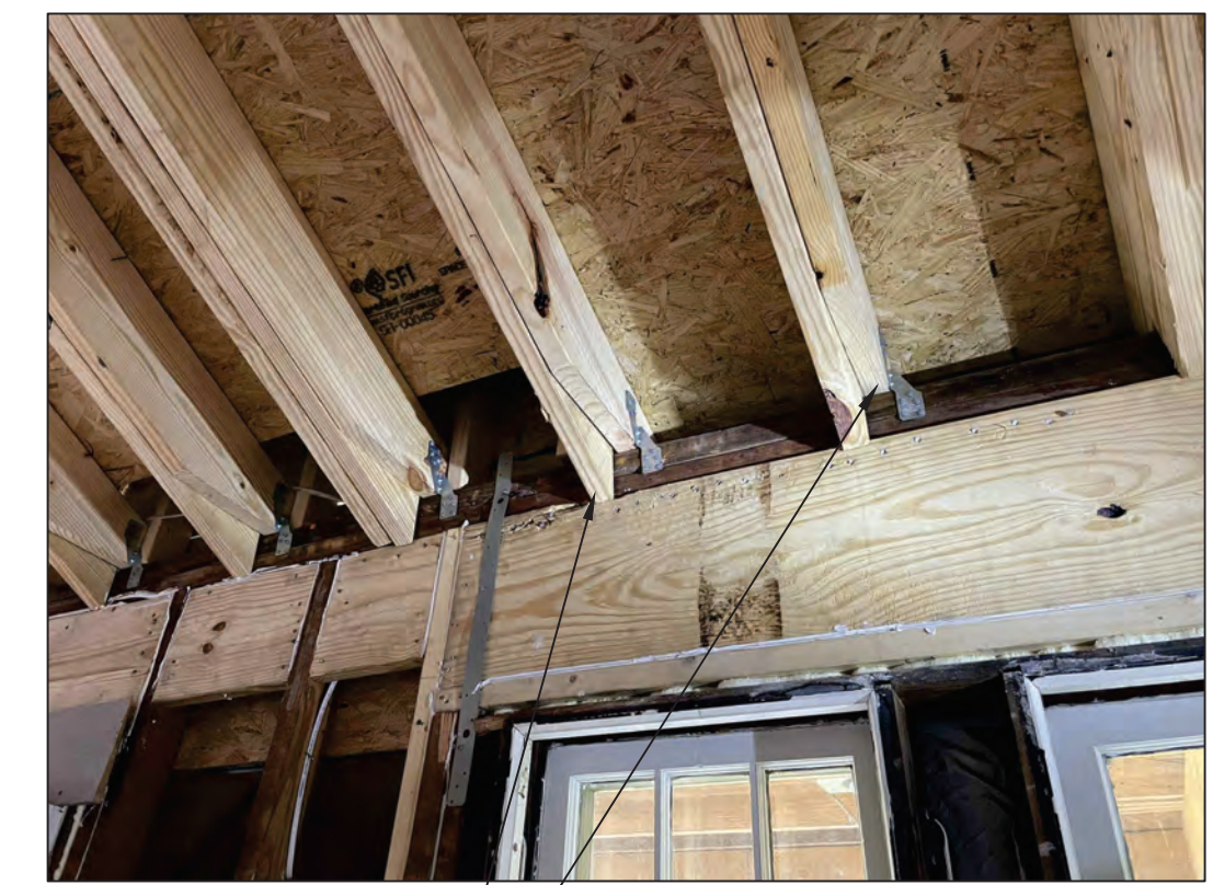
① Cuts on new rafters are more than D/4
