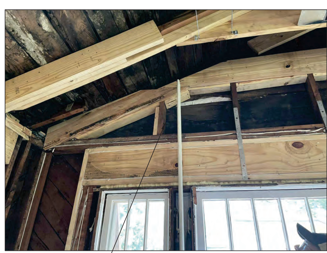
⑨1 No full height studs or bracing back to roof to support exterior bracket. See Photo 9.2
