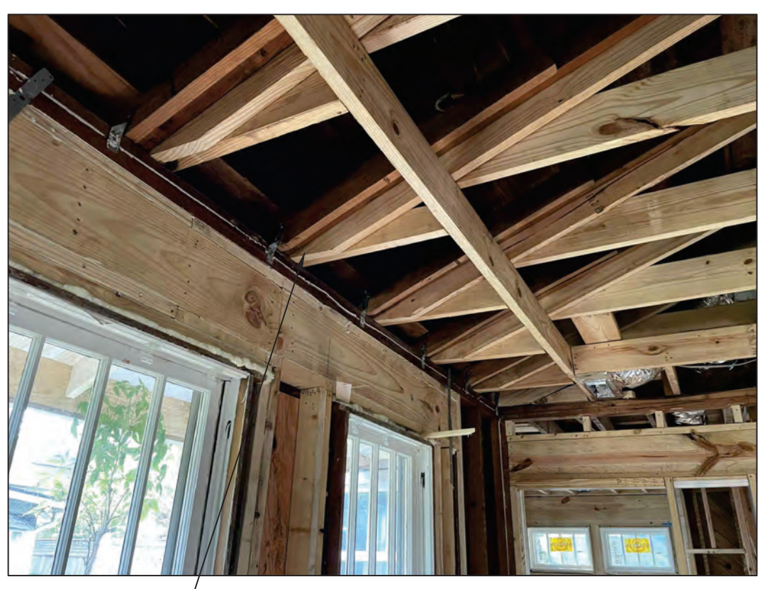
⑤ Cut on new rafters is more than D/4.
