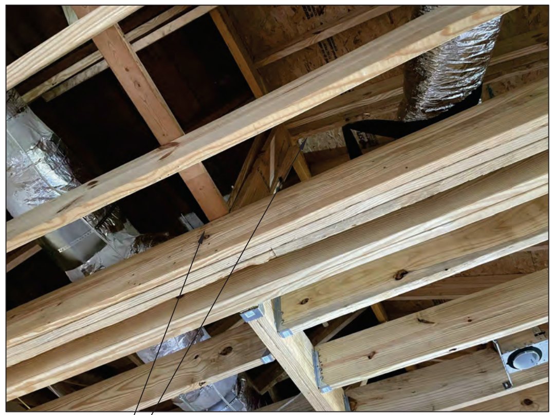
② New ridge beam is undersized and posted down to a triple ceiling joist.
