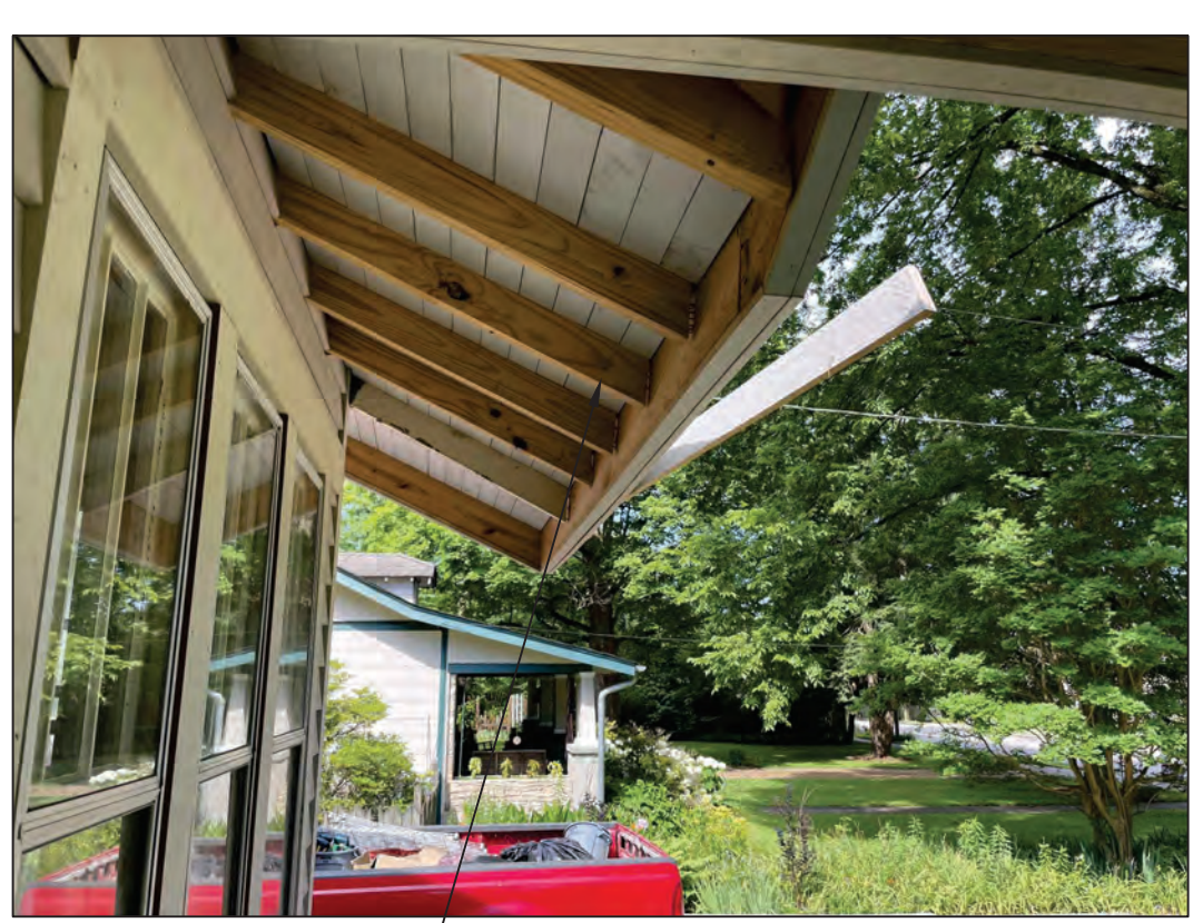
⑩ Rafter tails too short and therefore not properly tied to band. Use metal clip angles or joist hangers
