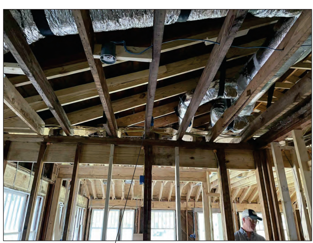
⑧ Ends of ceiling joist need to be blocked or a continuous lateral brace installed over the top.
