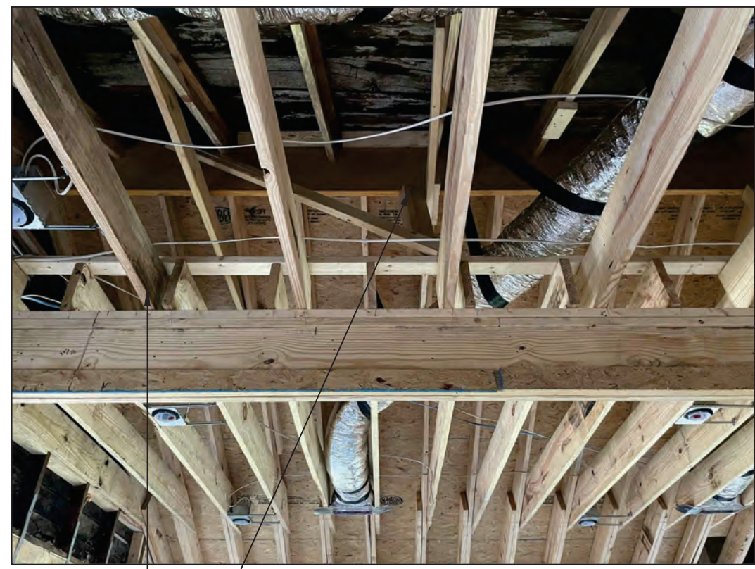
③ New ridge beam is improperly posted down at too sharp of an angle to a header that does not have enough capacity to support. End of ceiling joist are not aligned to develop roof thrust.
