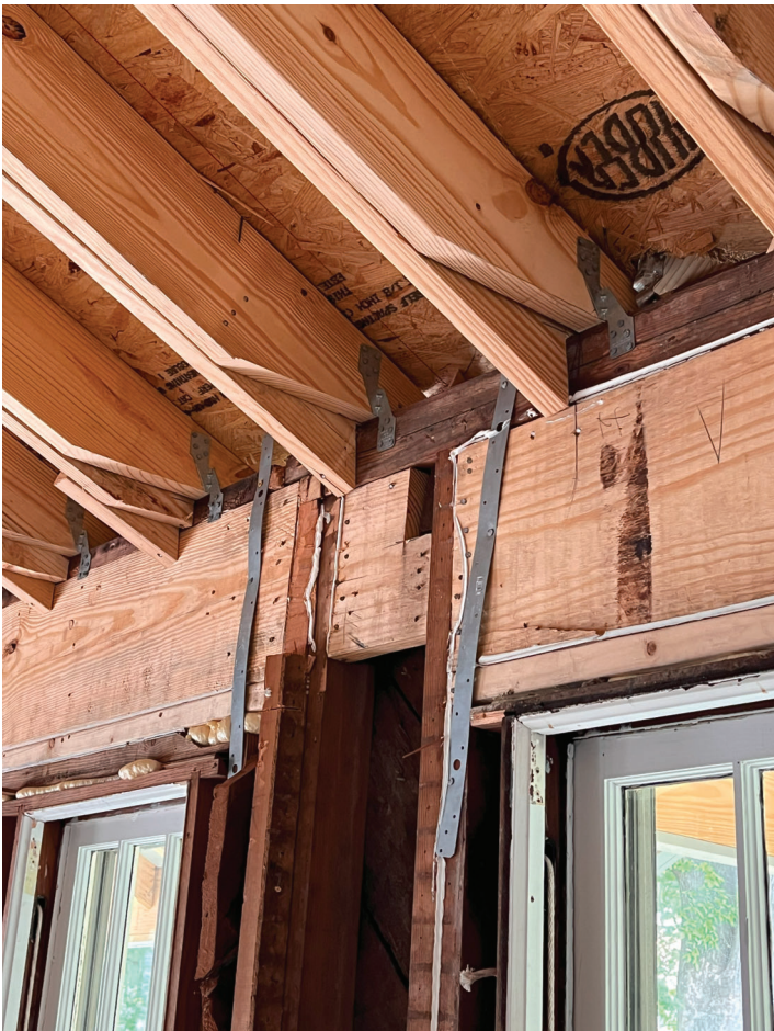
IMPROPER RAFTER CONSTRUCTION
