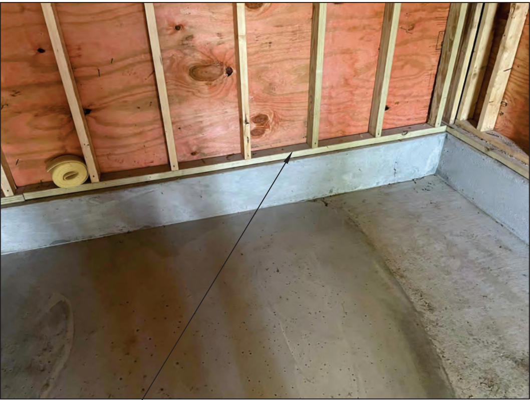
① No anchor rods between sill and foundation wall. Install 1/2" diameter x 5' Titen HDs at 32" oc.
