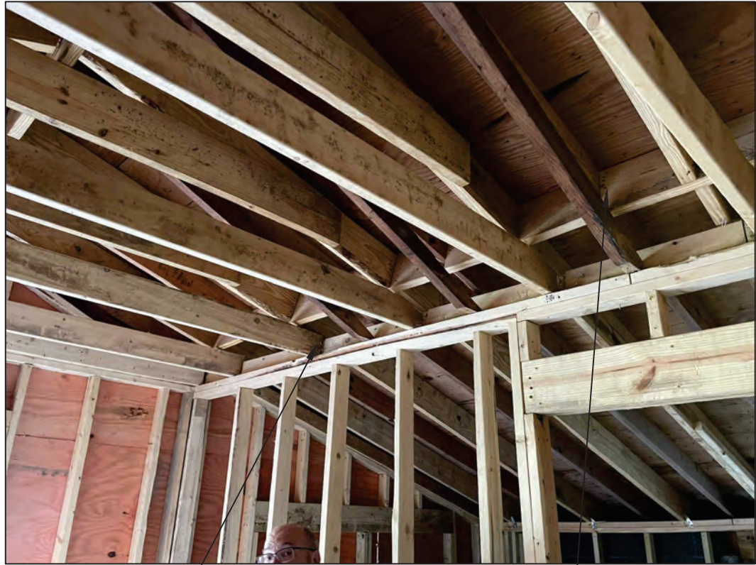
③ Improper connection of ceiling joists. Improper splicing and support of roof rafters.
