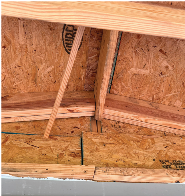
UNSUPPORTED PORCH ROOF CONSTRUCTION
