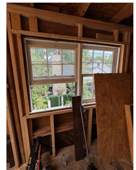
EXISTING NON-HISTORIC WINDOW CONDITIONS SHOW NEWER AGE OF FRAMING AND METAL JAMBS.
