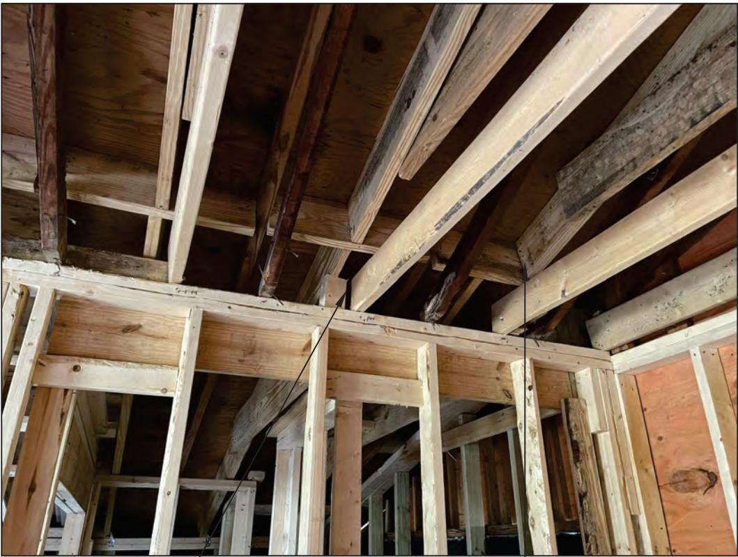
② Improper laps on ceiling joists. Improper splicing and support of roof rafters.
