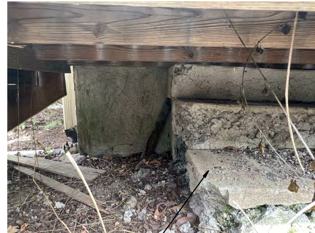
STAIRS UNDER EXISTING SIDE PORCH. INVESTIGATE CONDITION AFTER REMOVAL OF SIDE PORCH AND WORK WITH STAFF FOR REPAIR OR NEXT STEPS.
