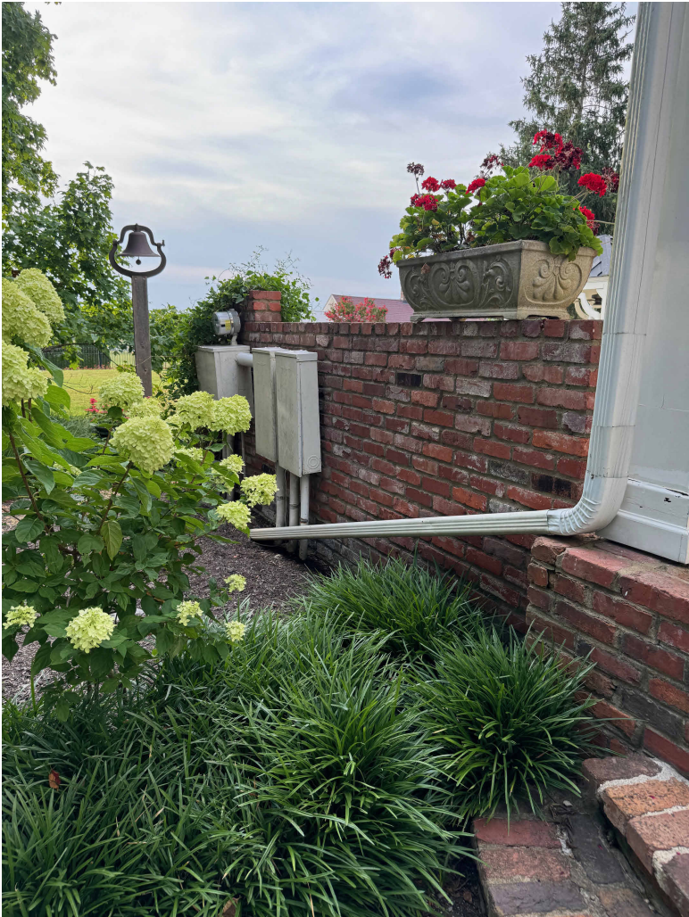
EXISTING ELECTRICAL METERS TO REMAIN
