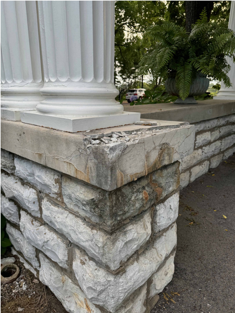
DAMAGE AT PORTE COCHERE
