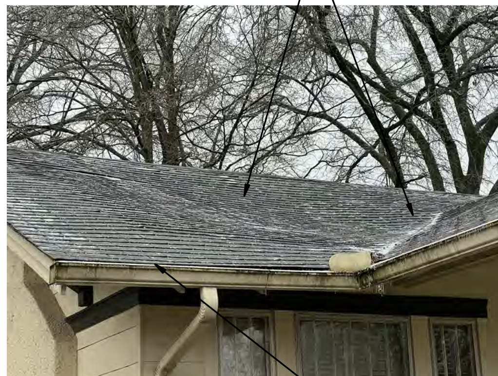
FRONT OF HOUSE, SHOWING STRUCTURAL SAG
