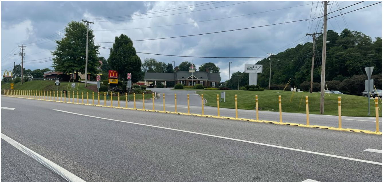
Figure 3 Example of Temporary Curbing with Delineators
