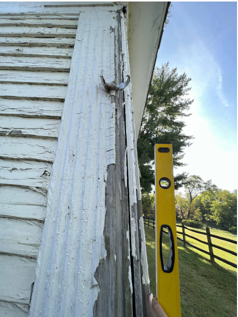
GARAGE SIDE REAR (OUT OF SQUARE)
