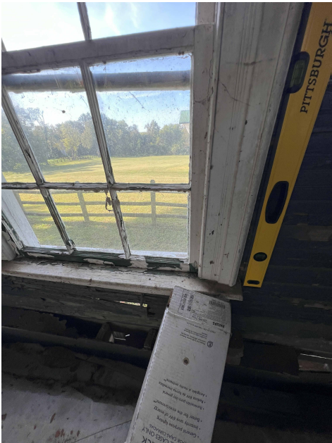
GARAGE INTERIOR WINDOW (OUT OF SQUARE)
