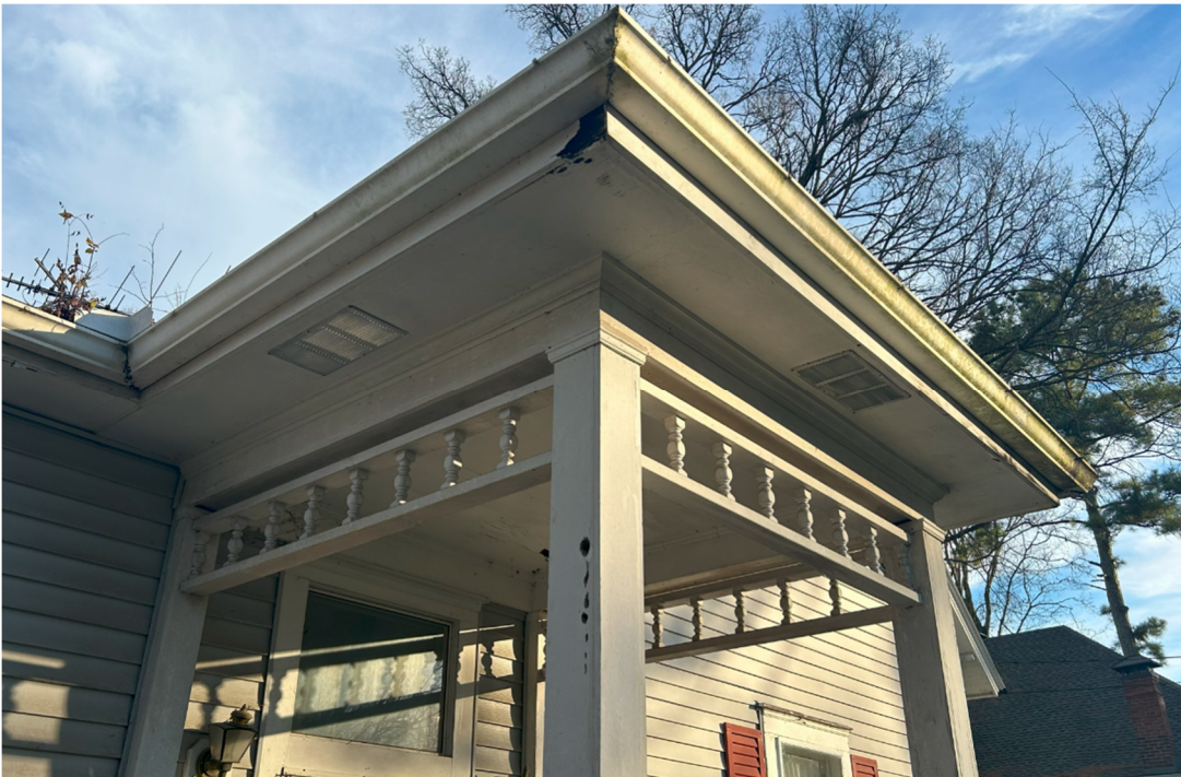
Image 7 - Porch has minimal detailing – overhead spindles are not original
