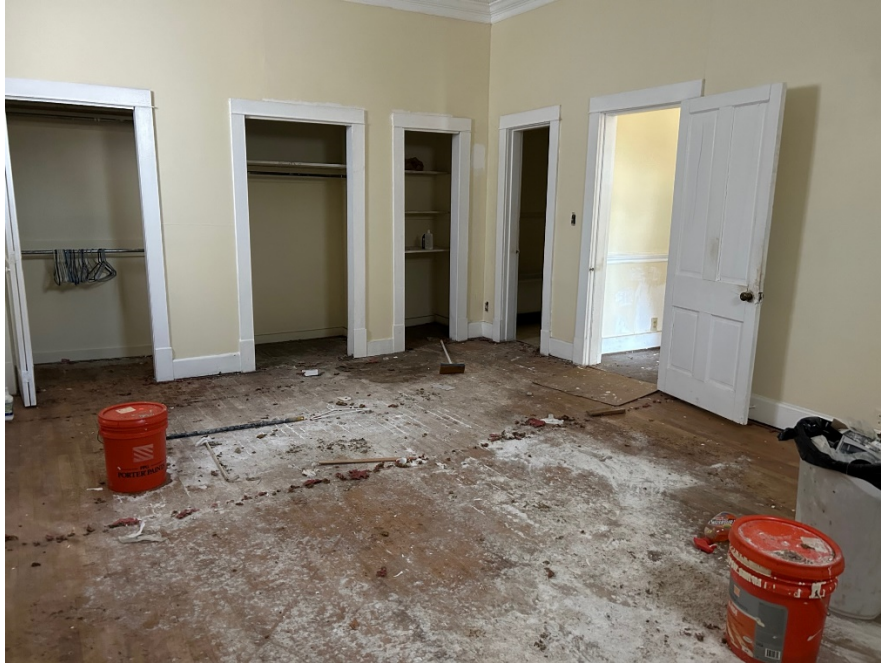
In this room a depression in the middle measured at 4" – 6" demonstrated a failure of the floor joists
