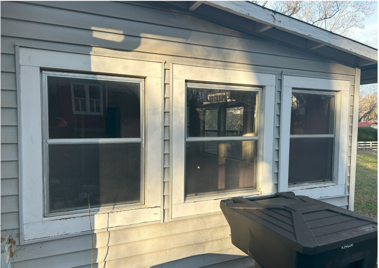
Image 11 - Windows at rear addition do not match vertical proportion of original windows and have no trim detail
