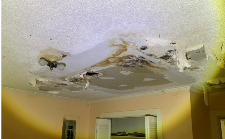
Significant water damage in the ceiling and sagging of 2" – 4" shows partial failure of ceiling structure
