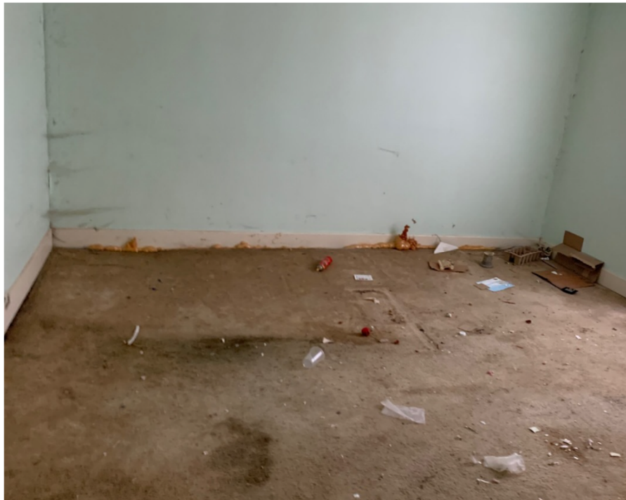
In this room a depression in the middle measured at 6" – 8" demonstrated a failure of the floor joists
