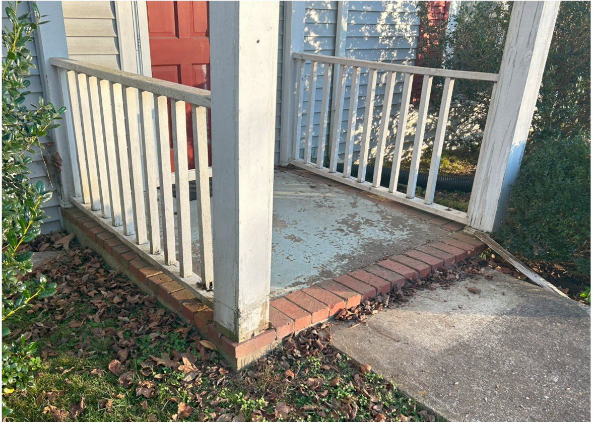
Images 8 & 9 - Porch railing is plain and not original – posts have begun to deteriorate at base
