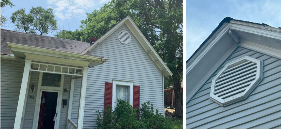
Images 5 & 6 - Front gable has minimal ornament – scrolled rafter extensions & octagonal vent which has been added and is not period appropriate
