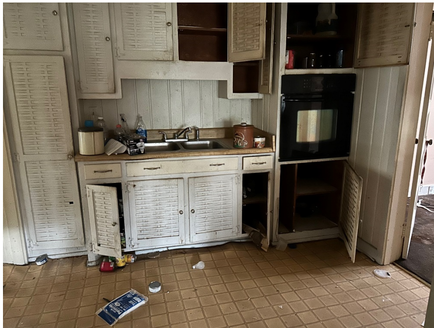
In this room a depression in the middle measured at 5" – 7" demonstrated a failure of the floor joists
