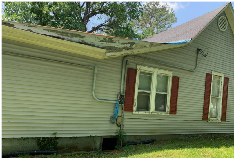
Image 15 - Severe deterioration to fascia where addition joins with original structure
