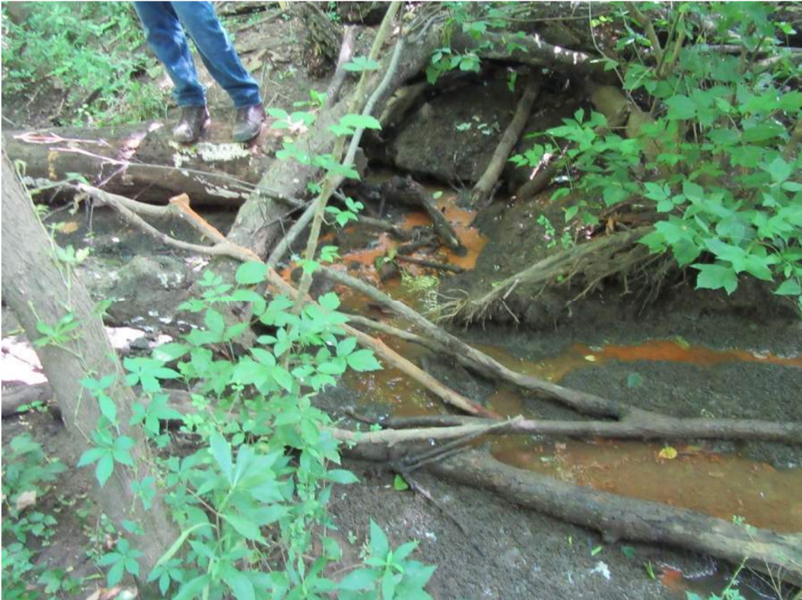
Photo No. 15: Seepage downstream of RCP pipe.
