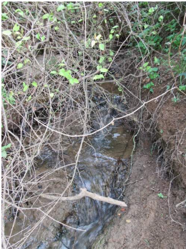
Photo No. 22: Seepage to left of spillway.
