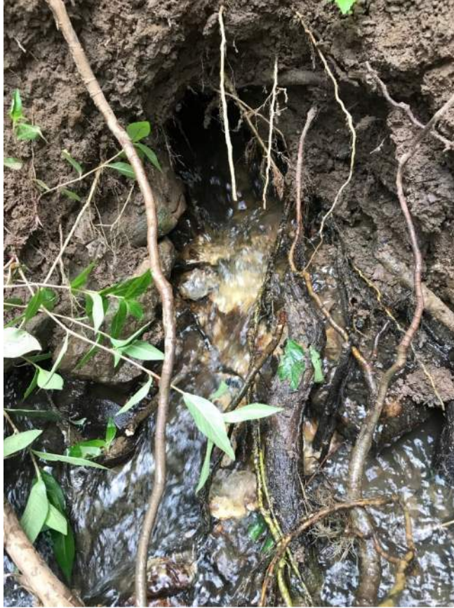
Photo No. 23: Seepage to left of spillway.
