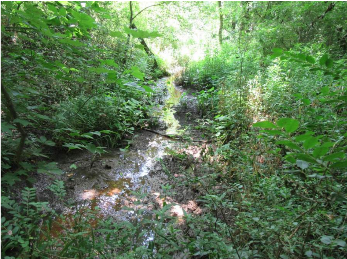
Photo No. 14: Seepage downstream of RCP pipe.
