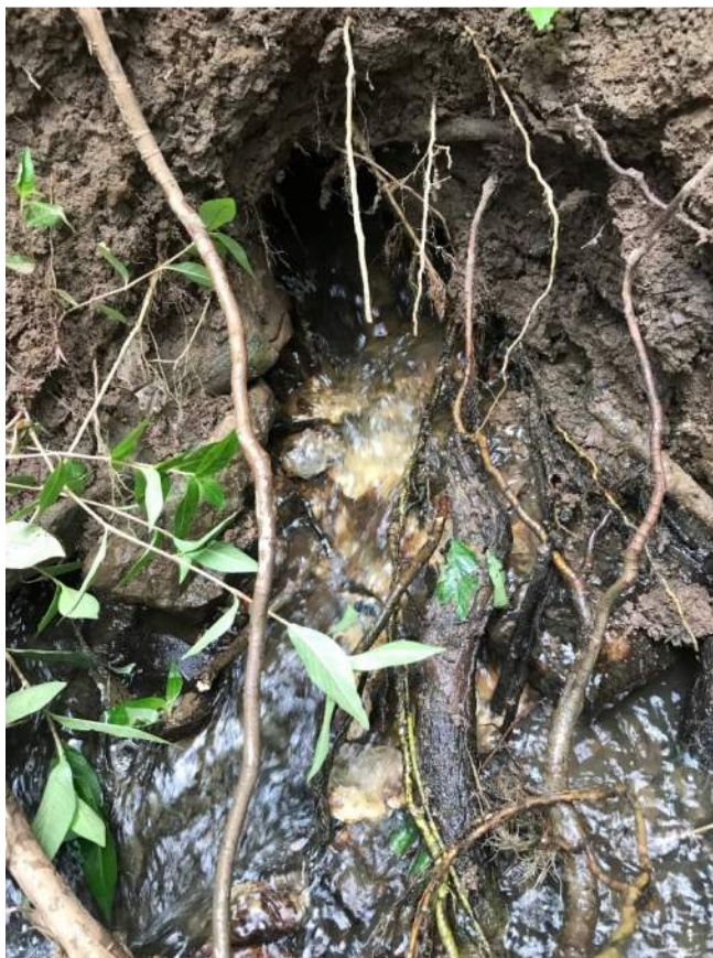
Photo No. 23: Seepage to left of spillway.
