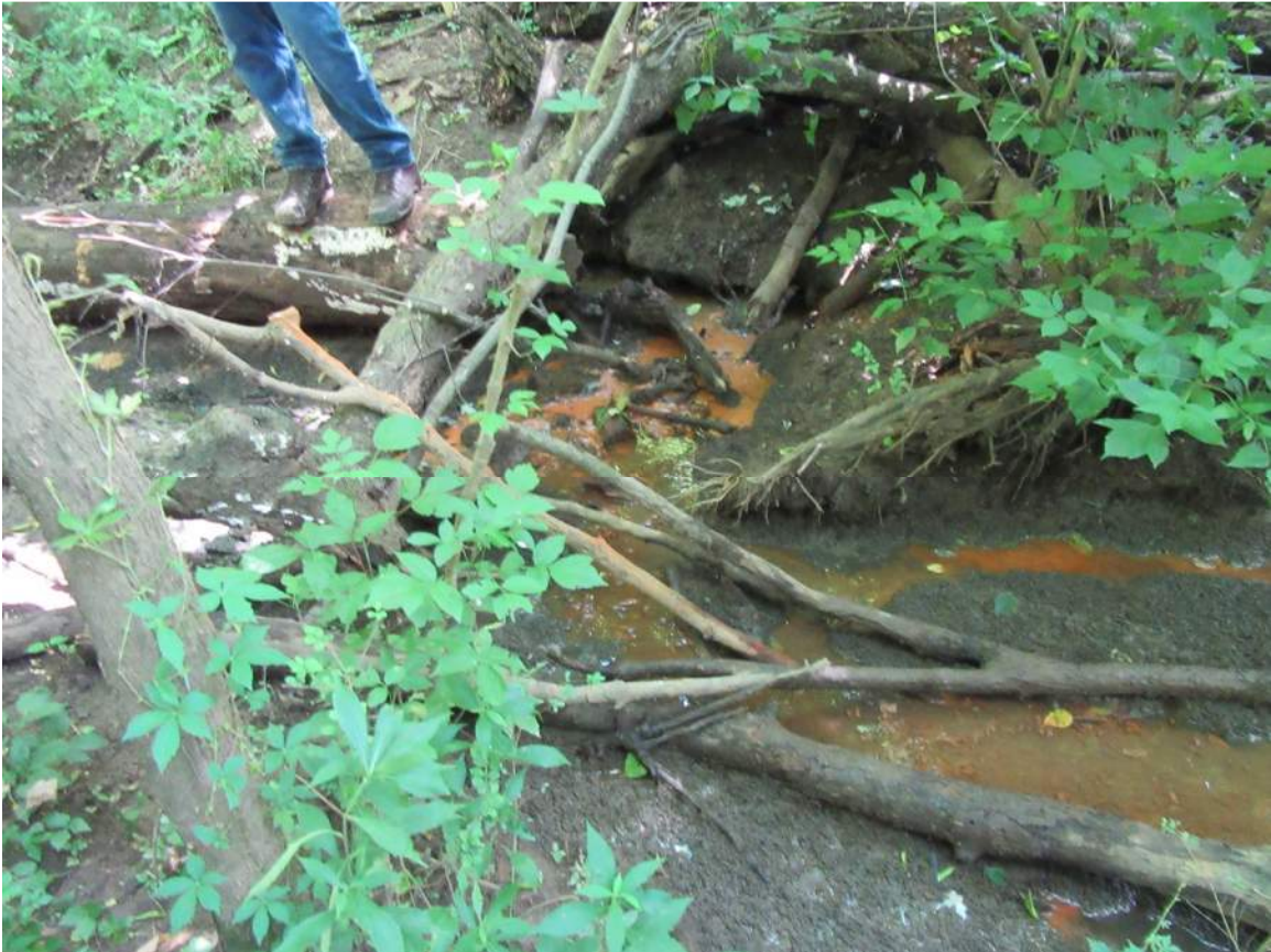
Photo No. 15: Seepage downstream of RCP pipe.
