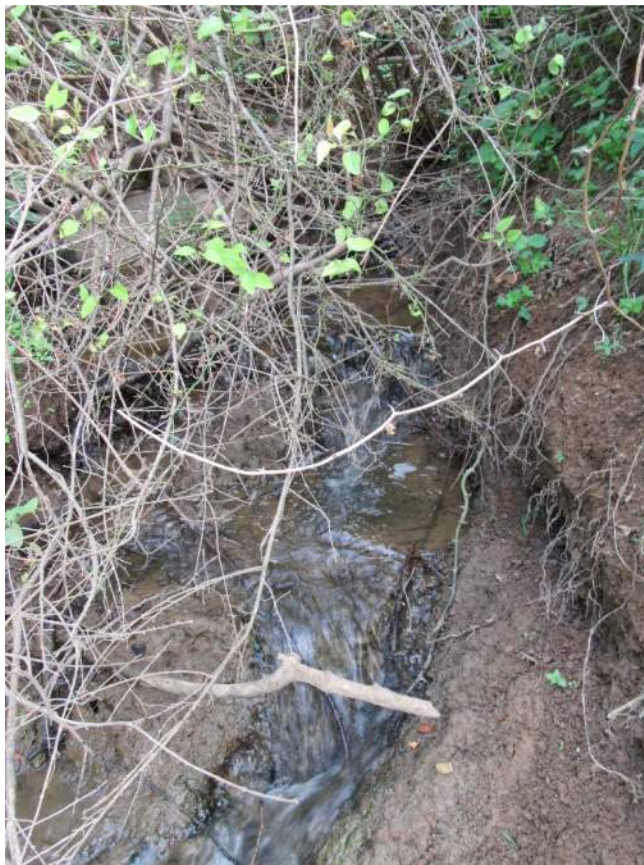
Photo No. 22: Seepage to left of spillway.
