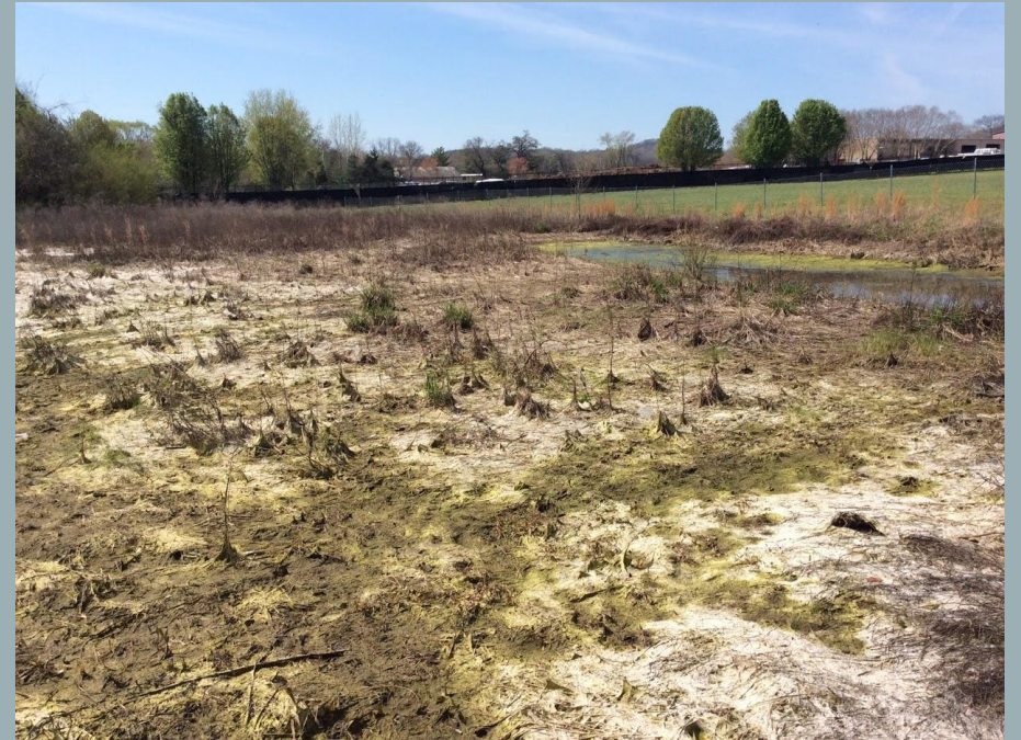
Public Works: Sand filter bed not installed
