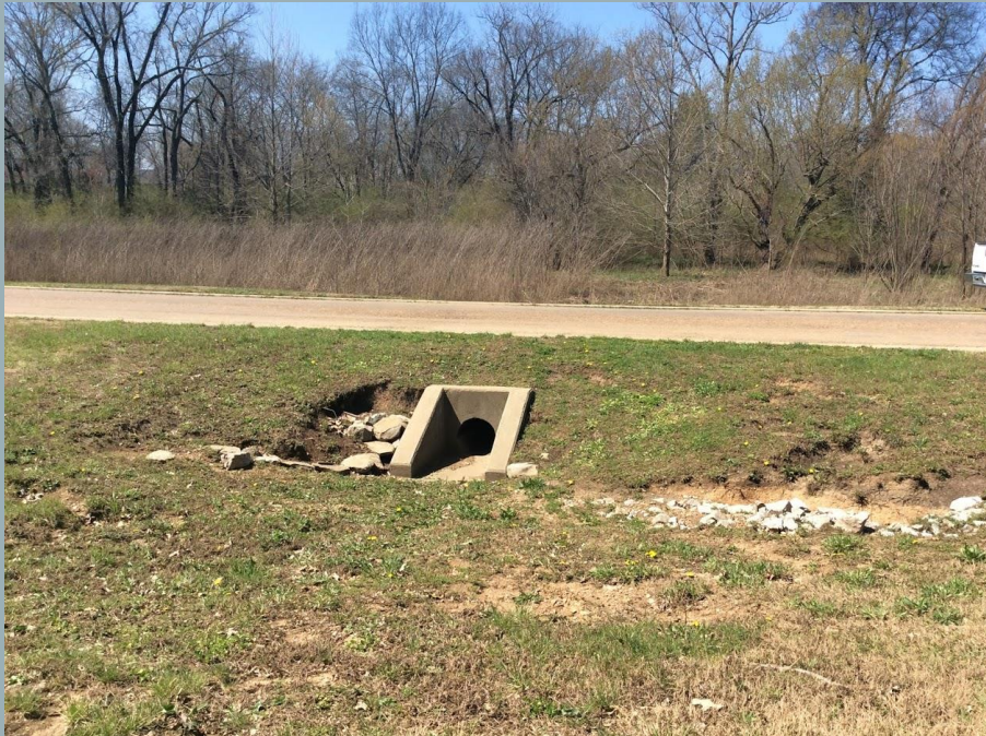
Eastern Flank: Fix erosion draining to stream
