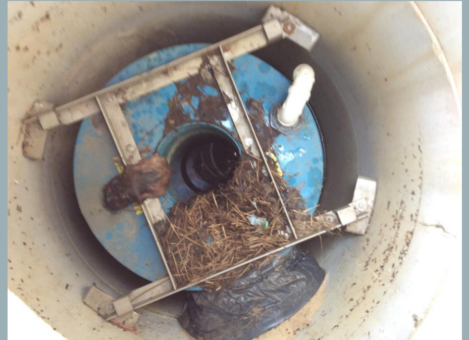
Fire Station #8: Clean water quality unit
