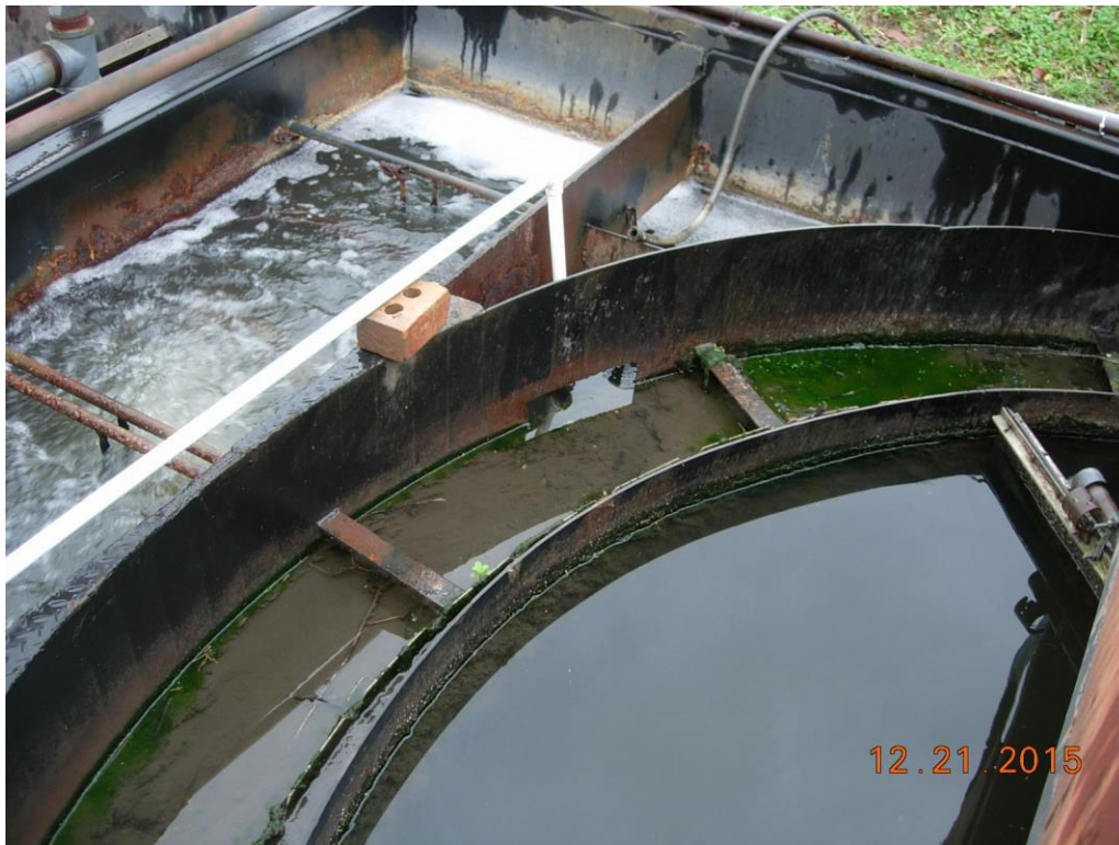
Clarifier with solids exiting weir trough
