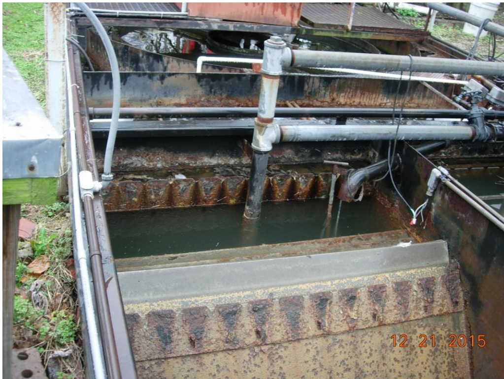
Corroded second filter structure & weir trough
