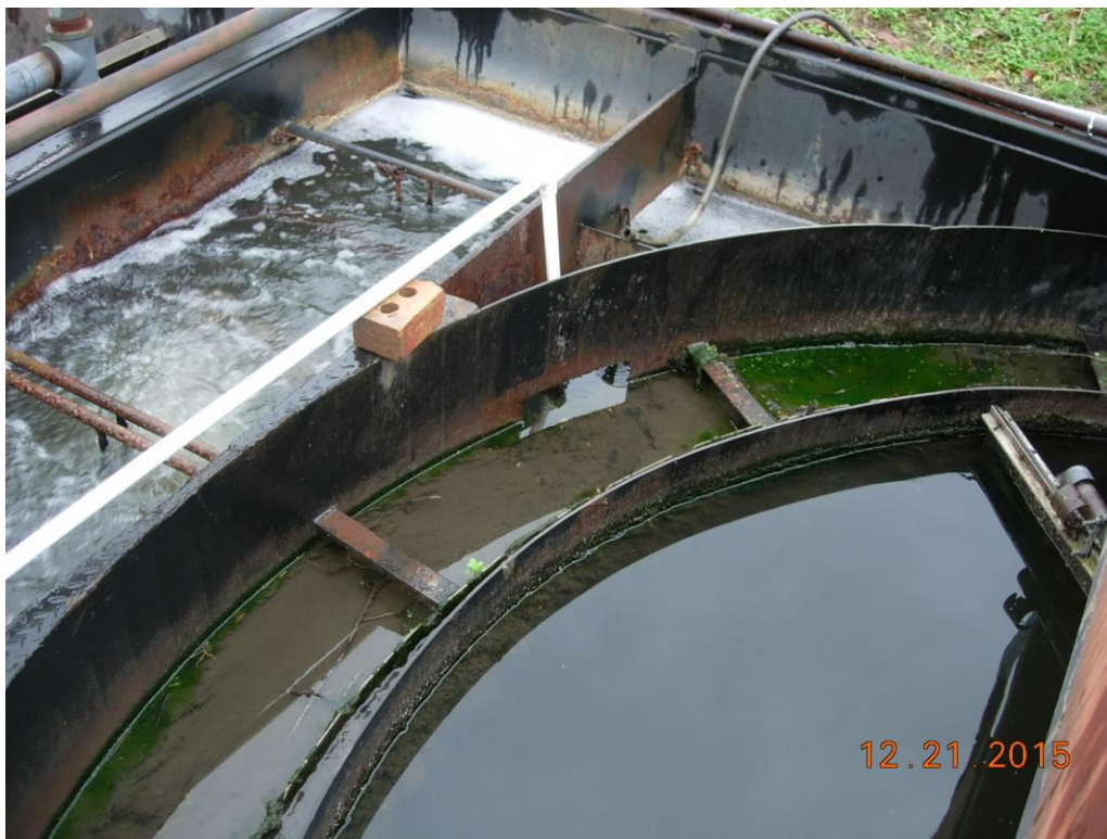
Clarifier with solids exiting weir trough
