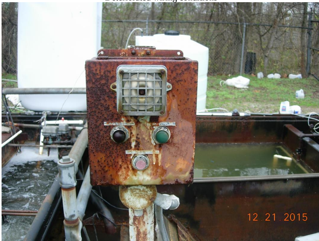
Deteriorated electrical system conditions
