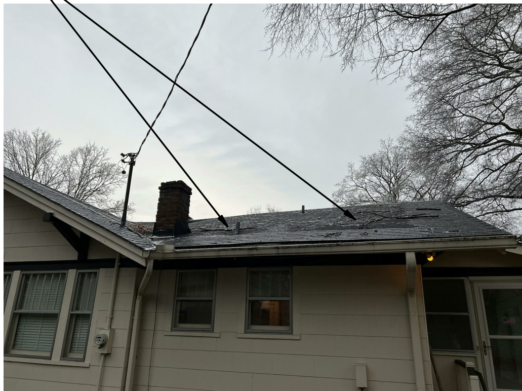
REAR OF HOUSE, SHOWING STRUCTURAL SAG
