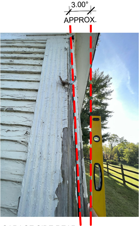
GARAGE SIDE REAR (OUT OF SQUARE)
