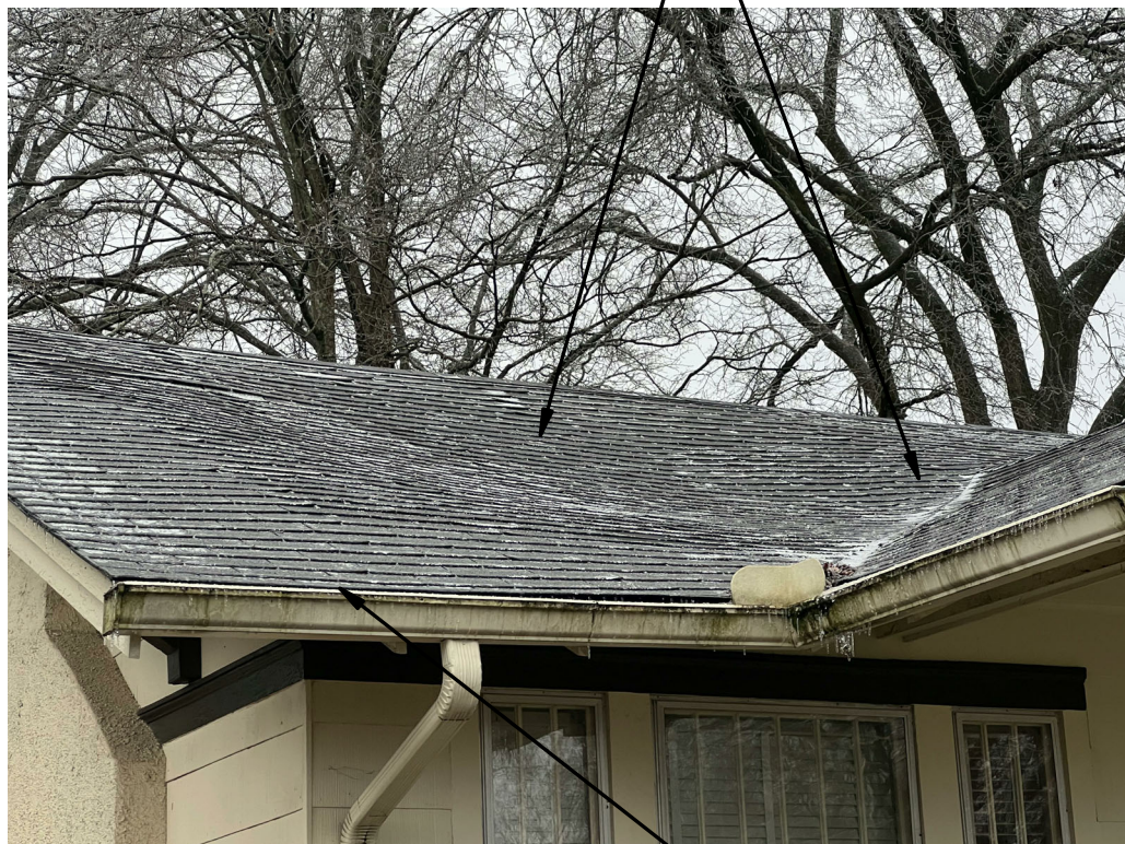
FRONT OF HOUSE, SHOWING STRUCTURAL SAG
