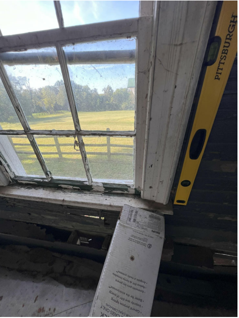
GARAGE INTERIOR WINDOW (OUT OF SQUARE)
