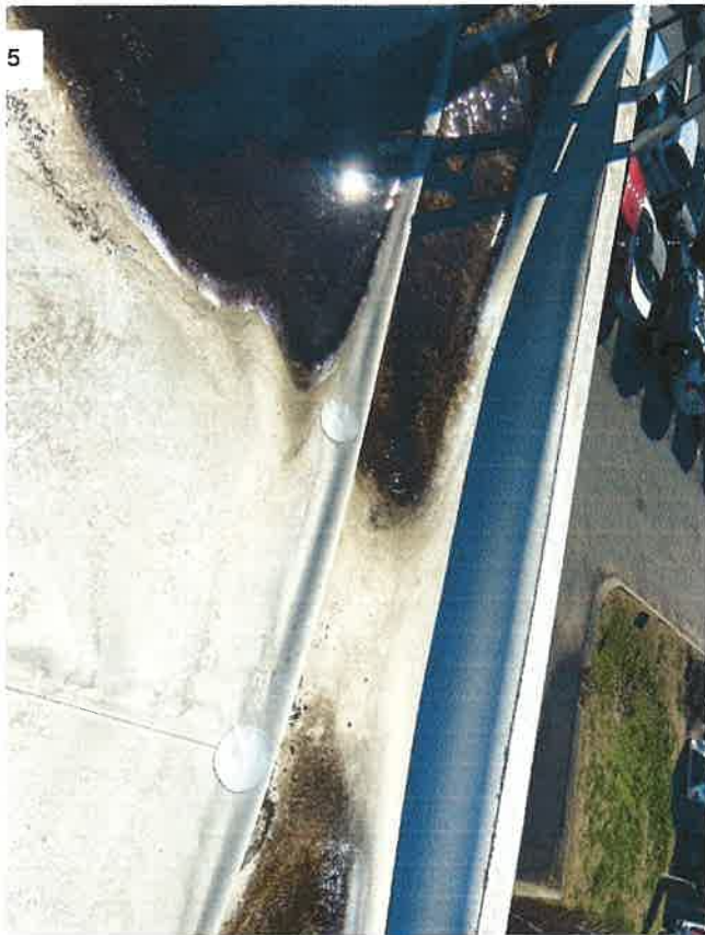
ponding water and wrinkled membrane
