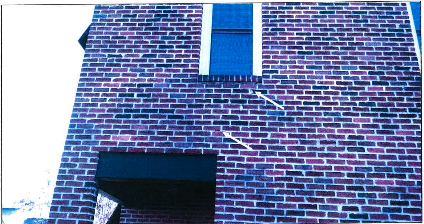
South (side) elevation of the building. Note crack in masonry above front entry porch.
