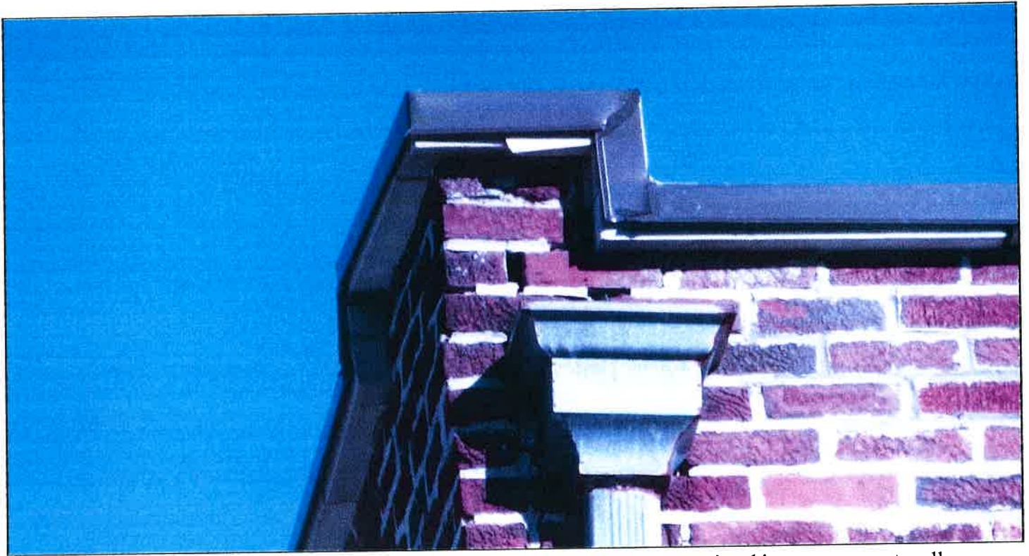
Open and missing mortar joints above downspout conductor head in west parapet wall.
