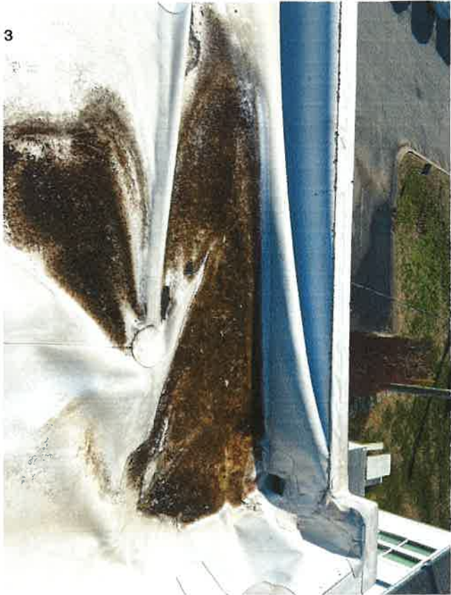
membrane loose from walls
