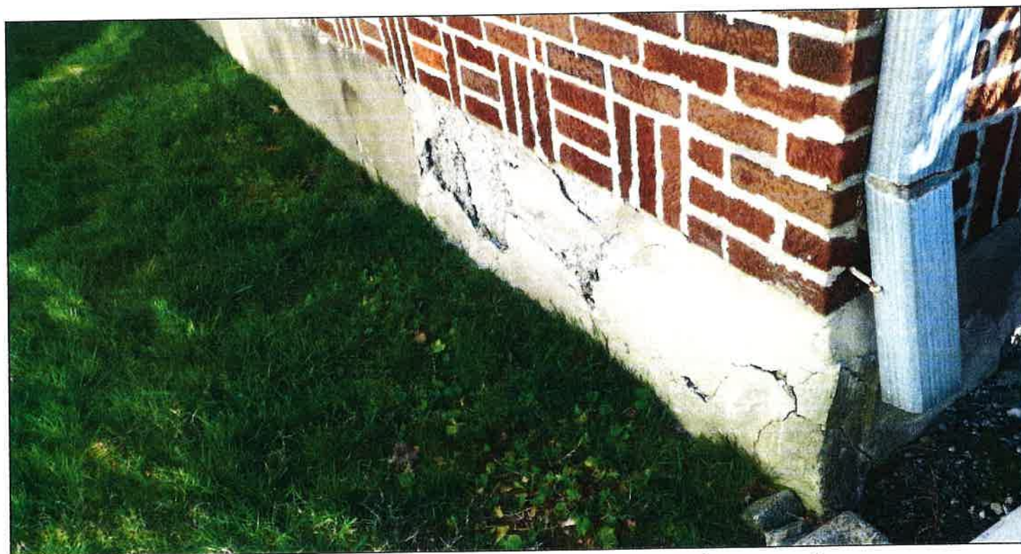
Cracked and spalled concrete on west elevation stem wall.
