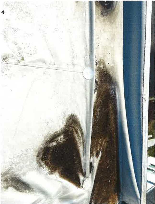
roof membrane loose and bridged
