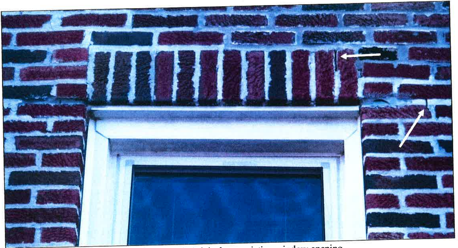
Cracks in brick above existing window opening.
