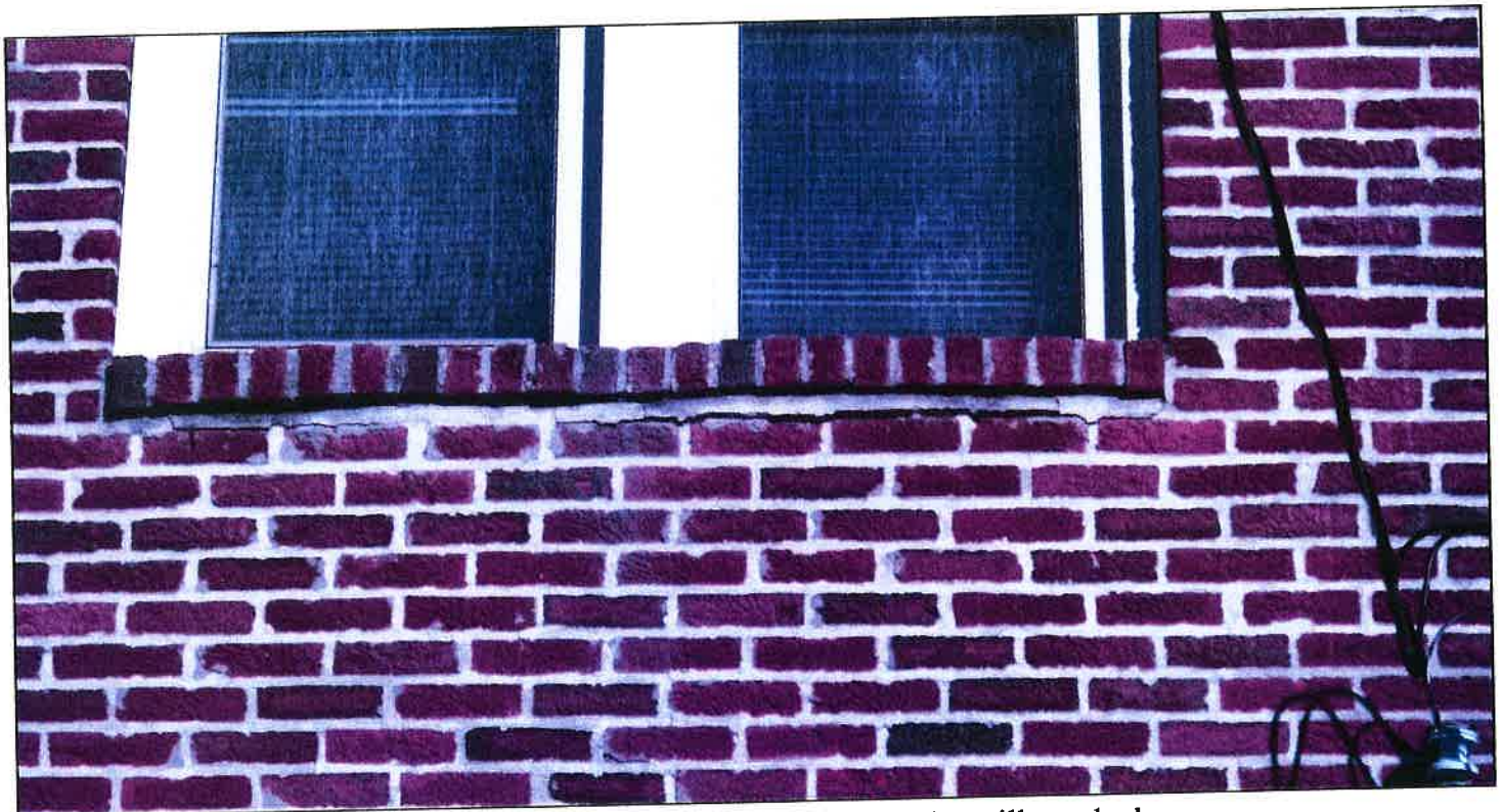
Crack in brick below existing window sill row lock.
