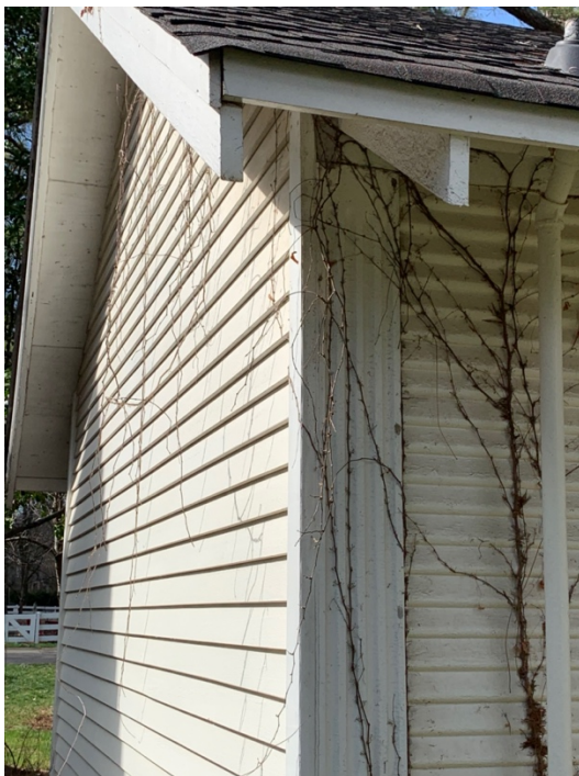
View of back side of the shed building showing new siding (2" w) juxtaposed against original siding (1" w)
