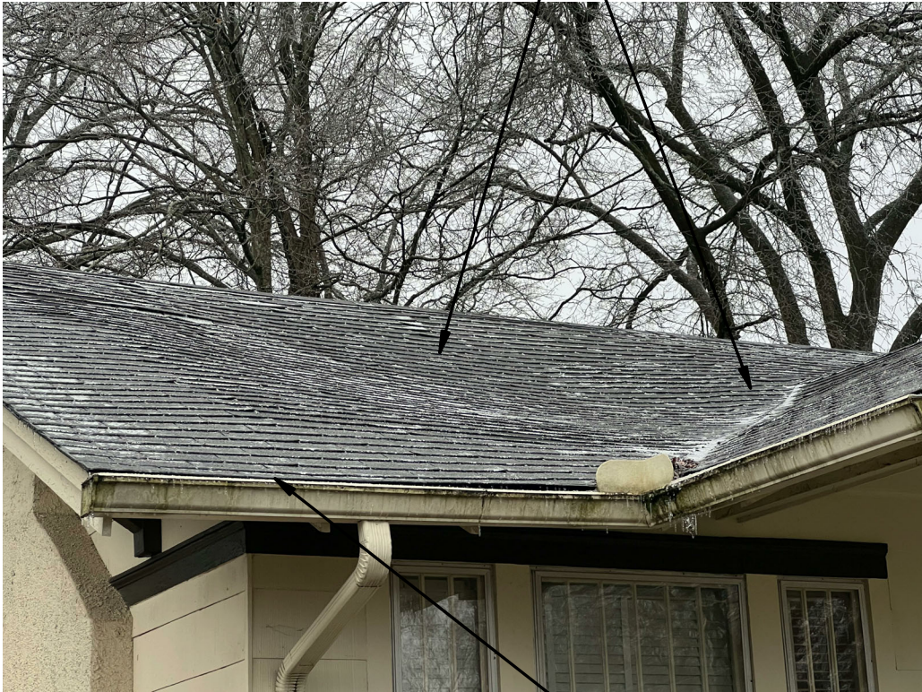
FRONT OF HOUSE, SHOWING STRUCTURAL SAG
