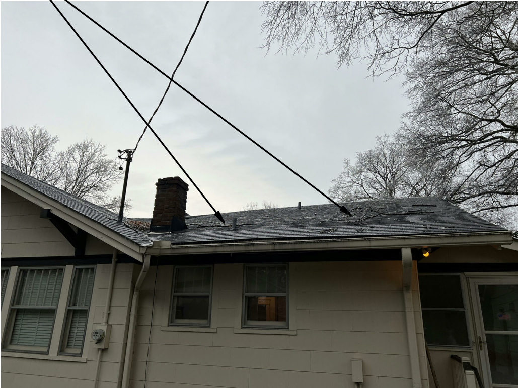
REAR OF HOUSE, SHOWING STRUCTURAL SAG
