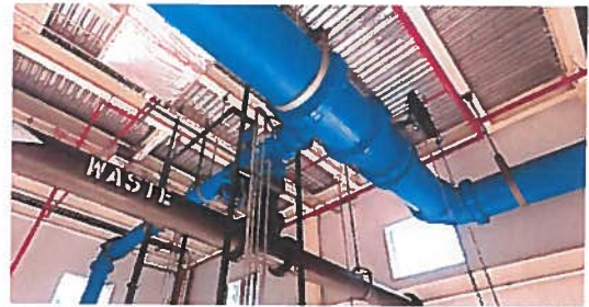
Figure 1 - Franklin WTP Valve Access Area
