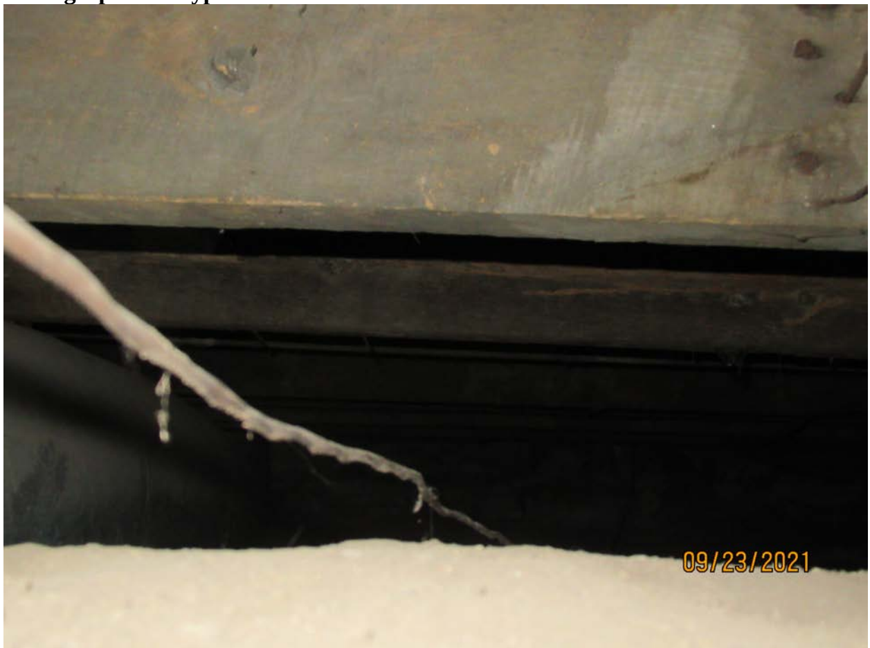
Photograph 95: Typical insect tunnels.
