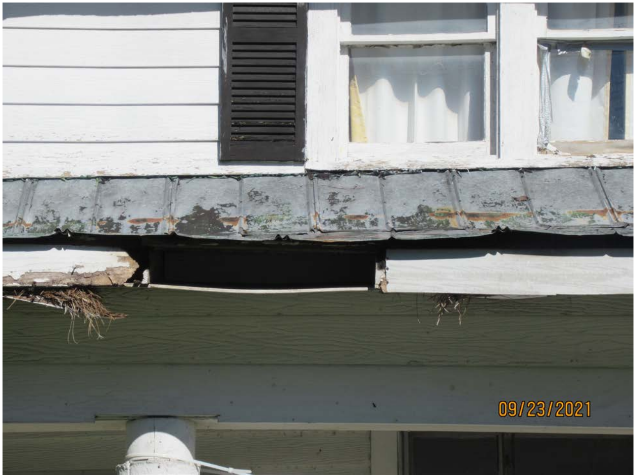
Photograph 3: Close-up of missing gutter board at front porch.
