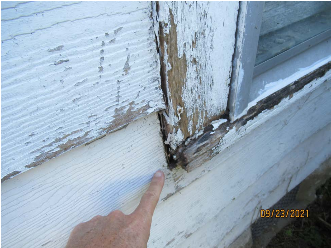
Photograph 29: Rotten wood trim at left-side wall.
