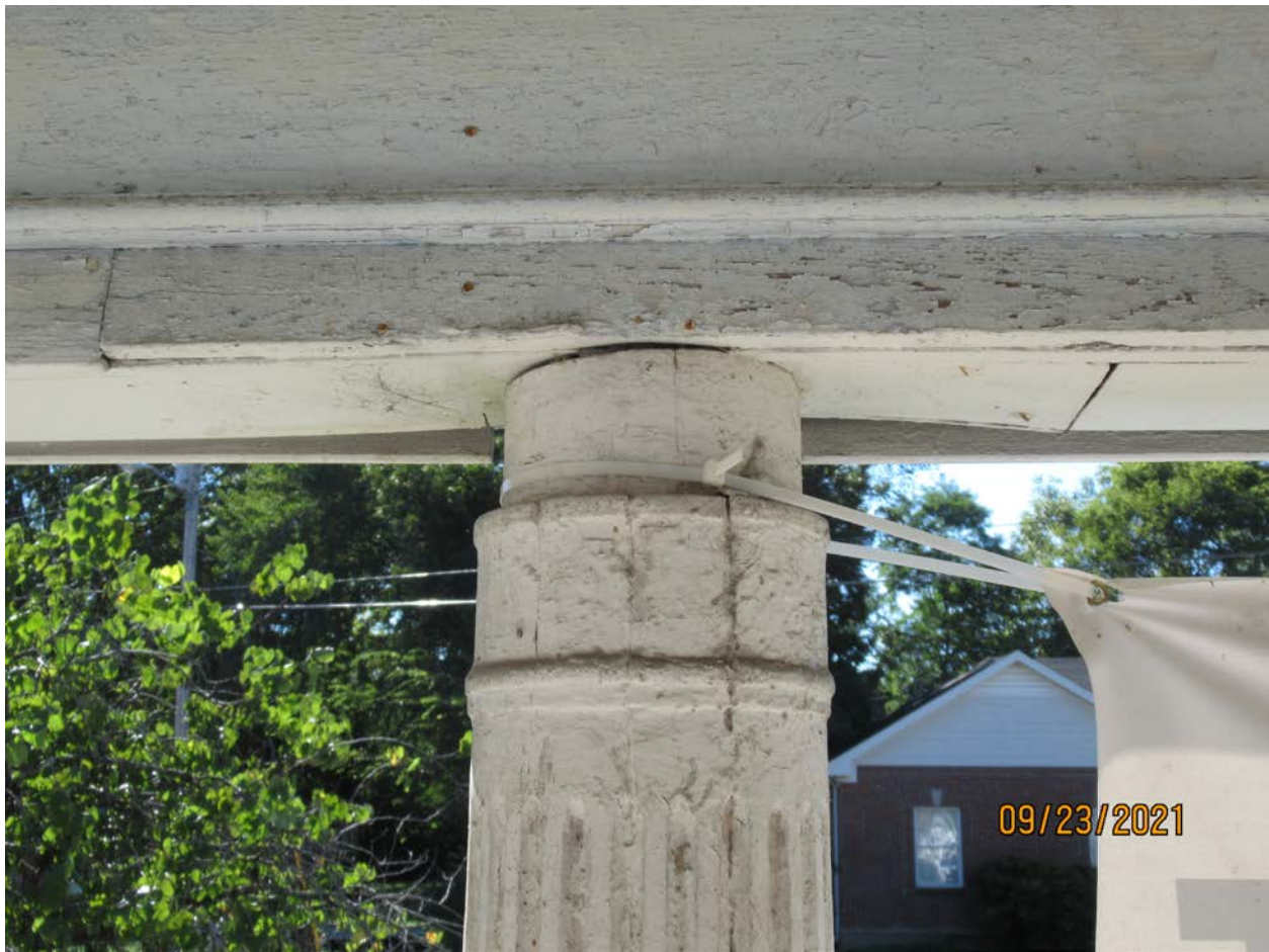
Photograph 9: Missing column capital at front porch.
