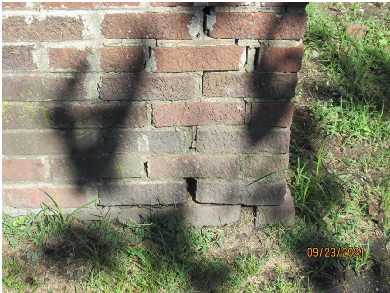
Photograph 11: Missing mortar at front porch columns.
