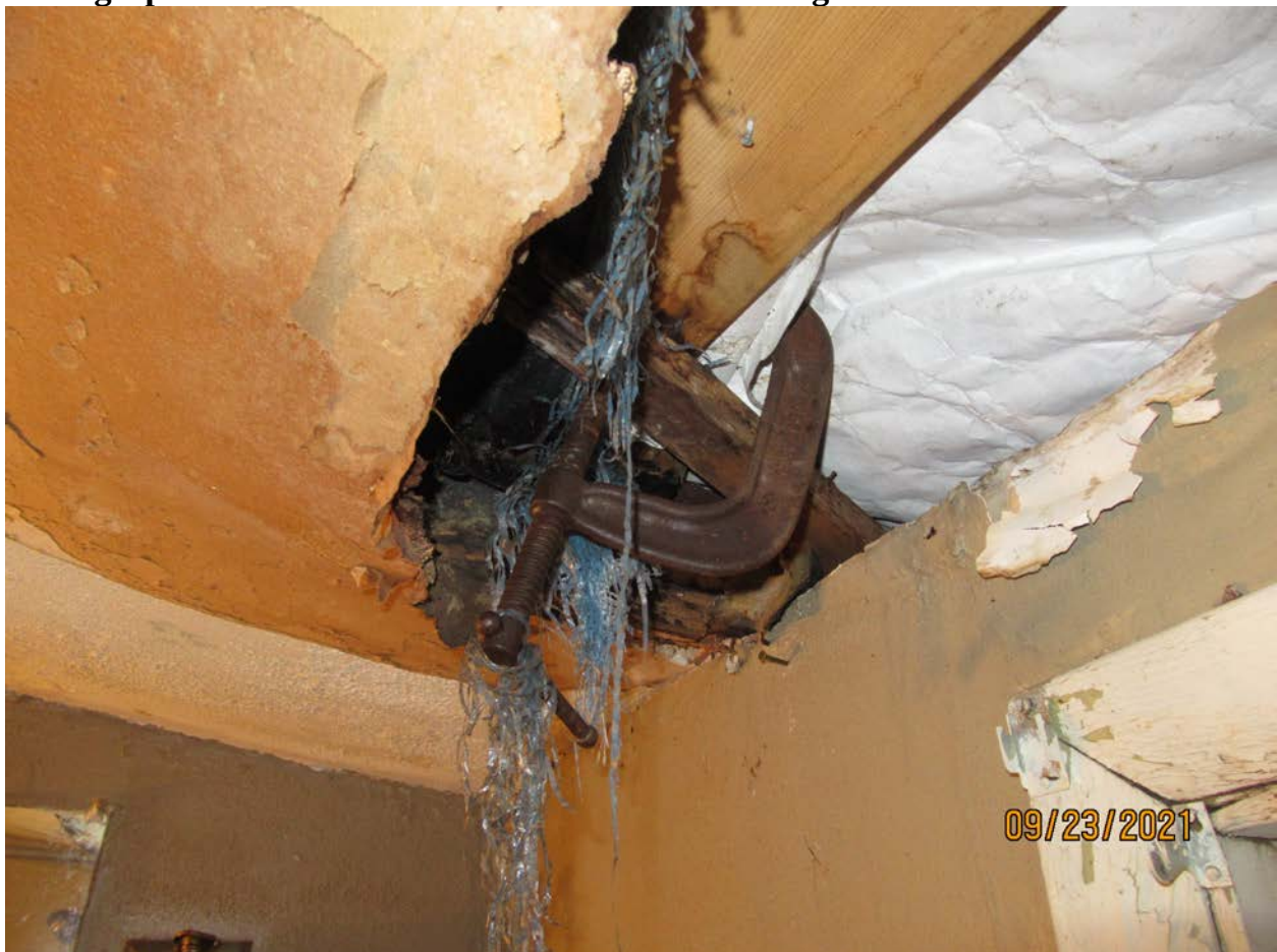
Photograph 65: View of second floor bathroom ceiling
