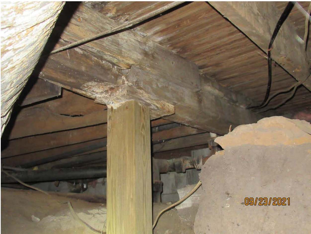
Photograph 96: Typical deteriorated roof framing.
