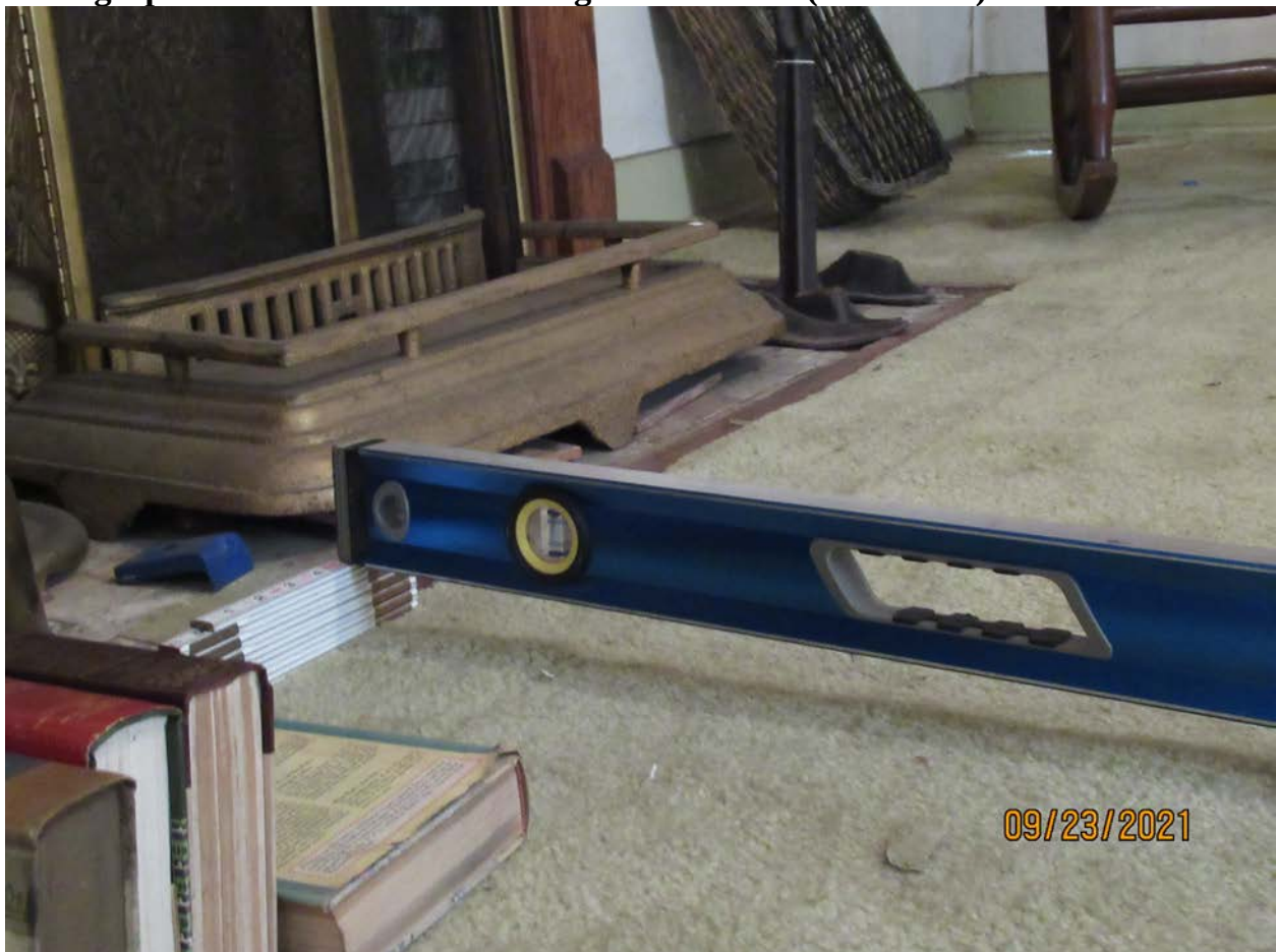
Photograph 39: Out-of-flat floor at right front room (main floor).
