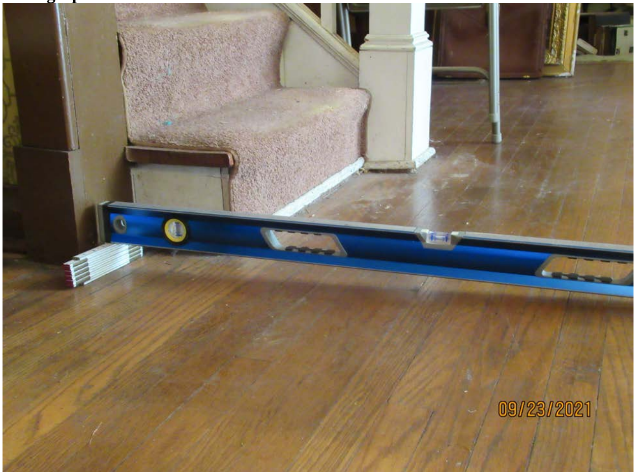
Photograph 35: Out-of-flat floor at stairwell.
