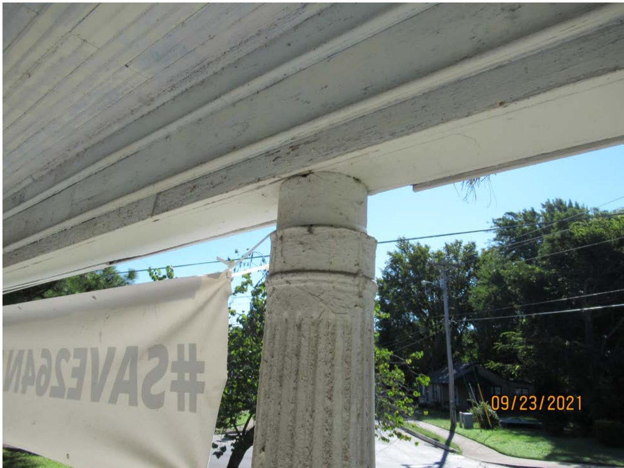
Photograph 7: Missing column capital at front porch.
