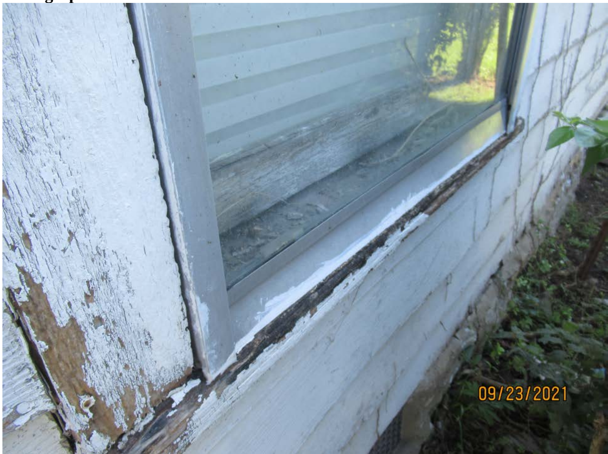
Photograph 30: Rotten wood trim at left-side wall.
