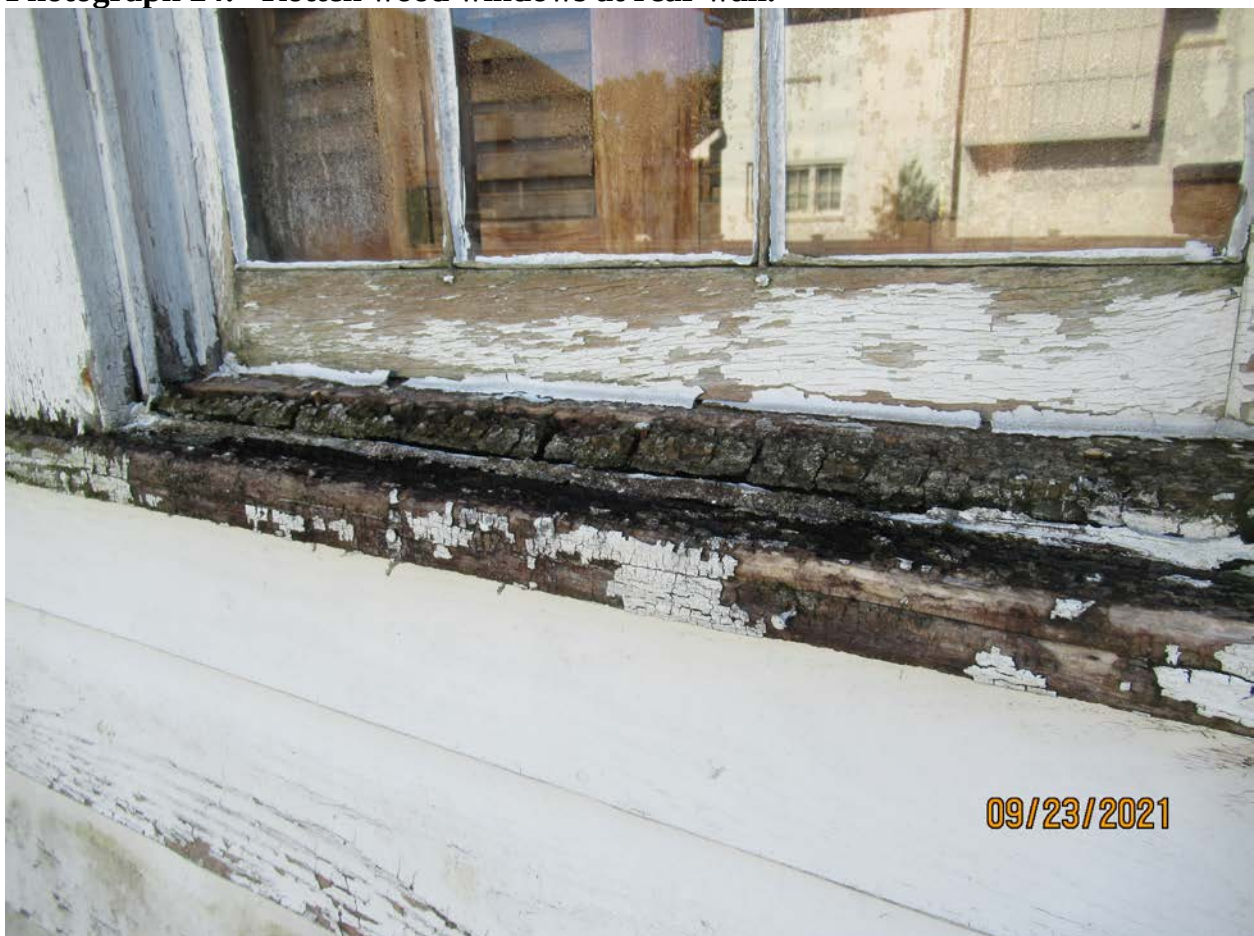
Photograph 24: Rotten wood windows at rear wall.
