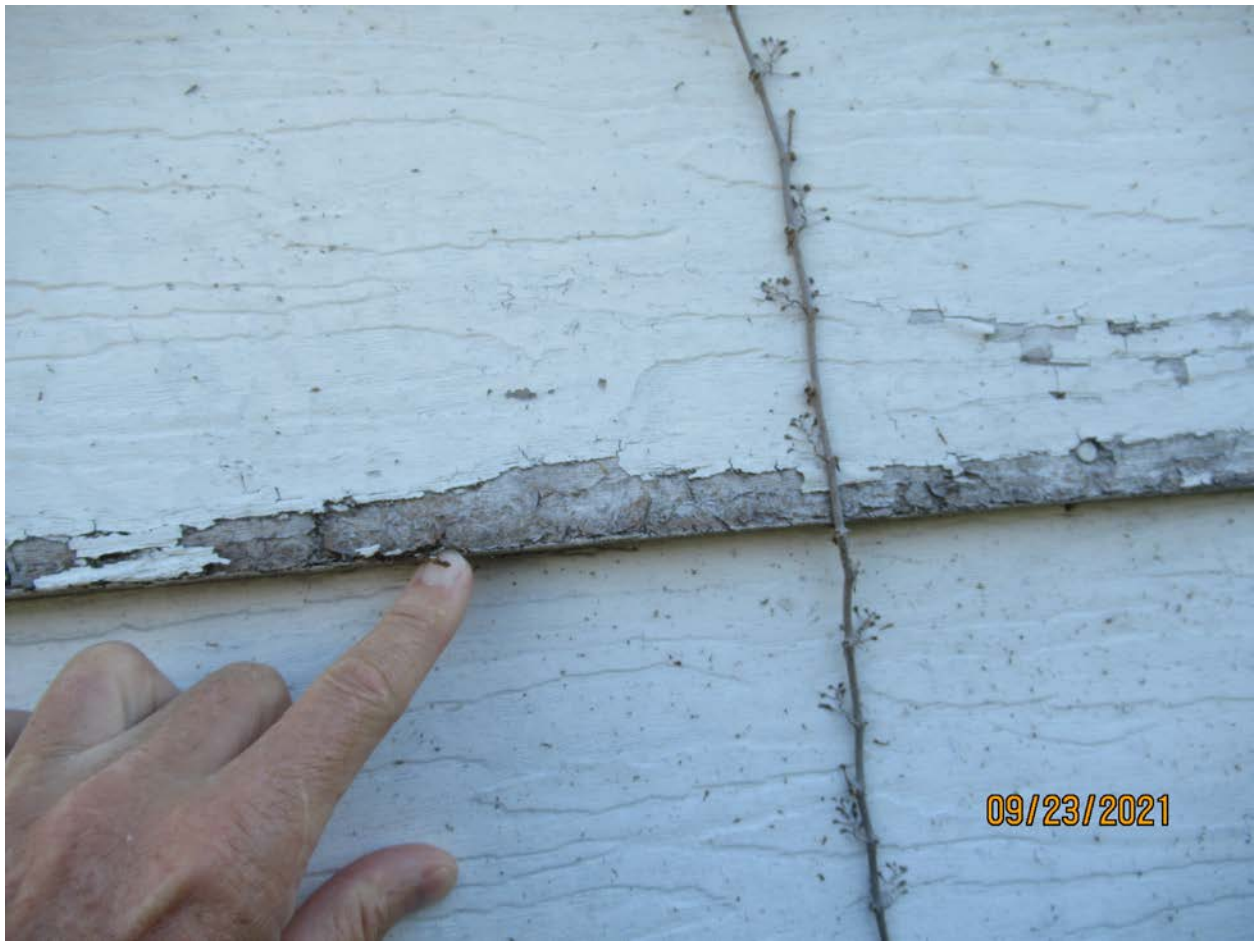
Photograph 31: Deteriorated siding at left-side wall.
