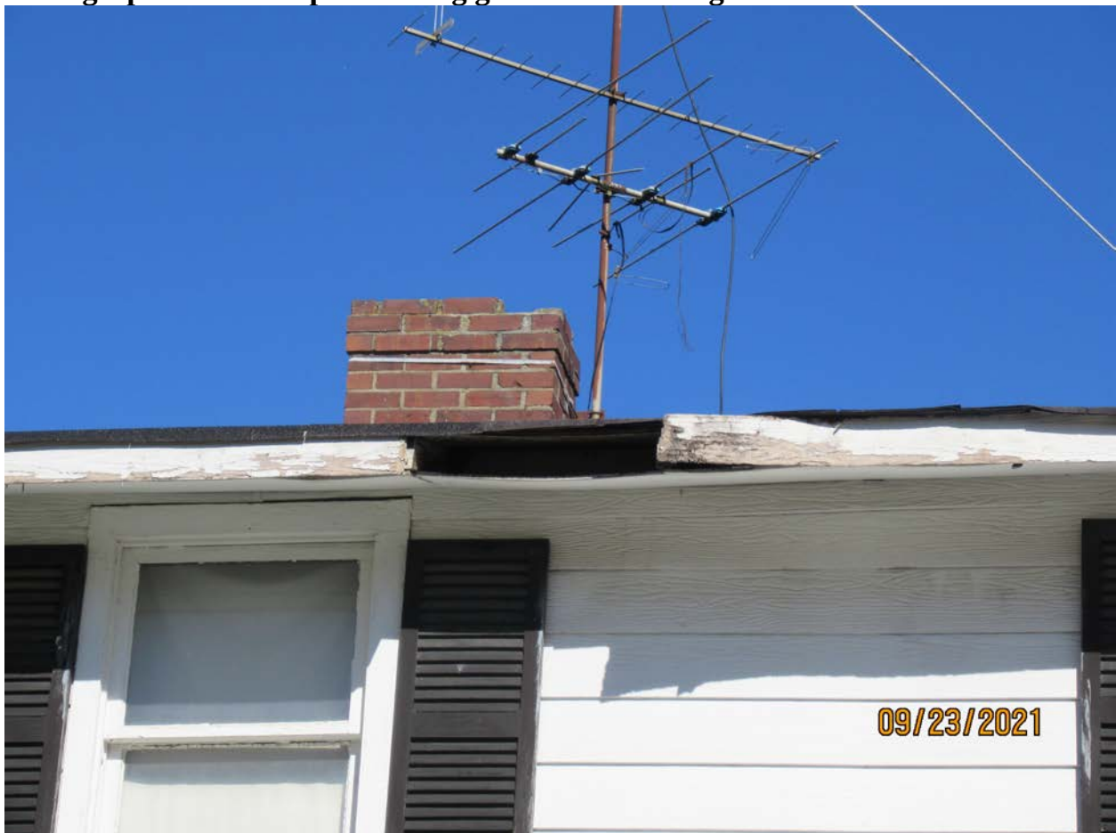
Photograph 2: Close-up of missing gutter board at high roof.
