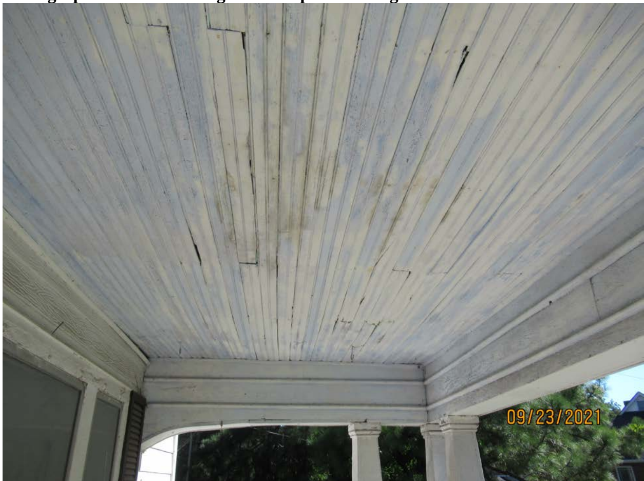
Photograph 8: Water damage to front porch ceiling.
