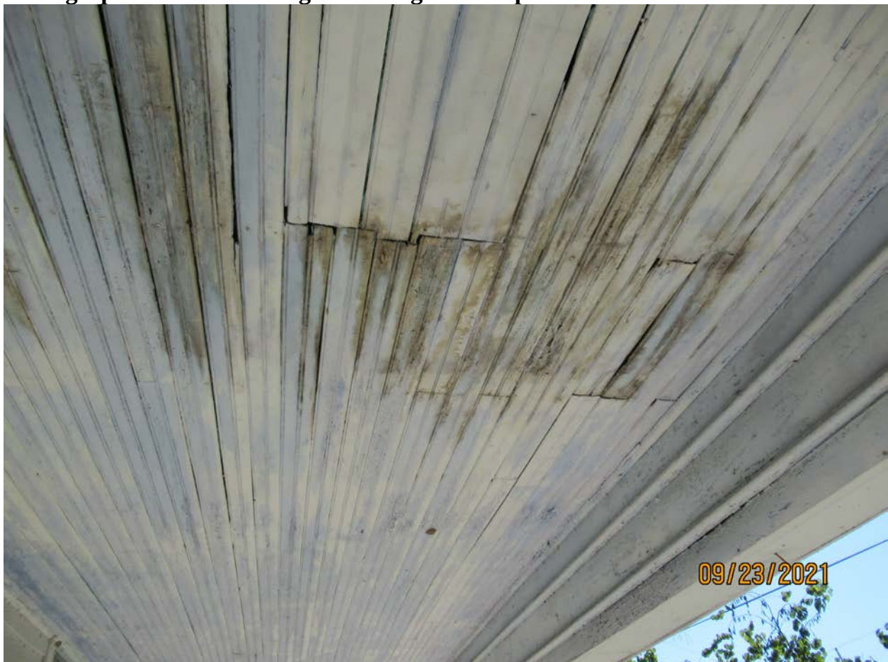
Photograph 6: Water damage to ceiling of front porch.
