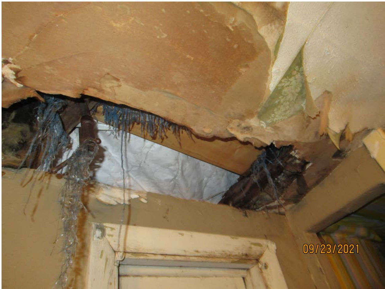
Photograph 64: View of second floor bathroom ceiling.
