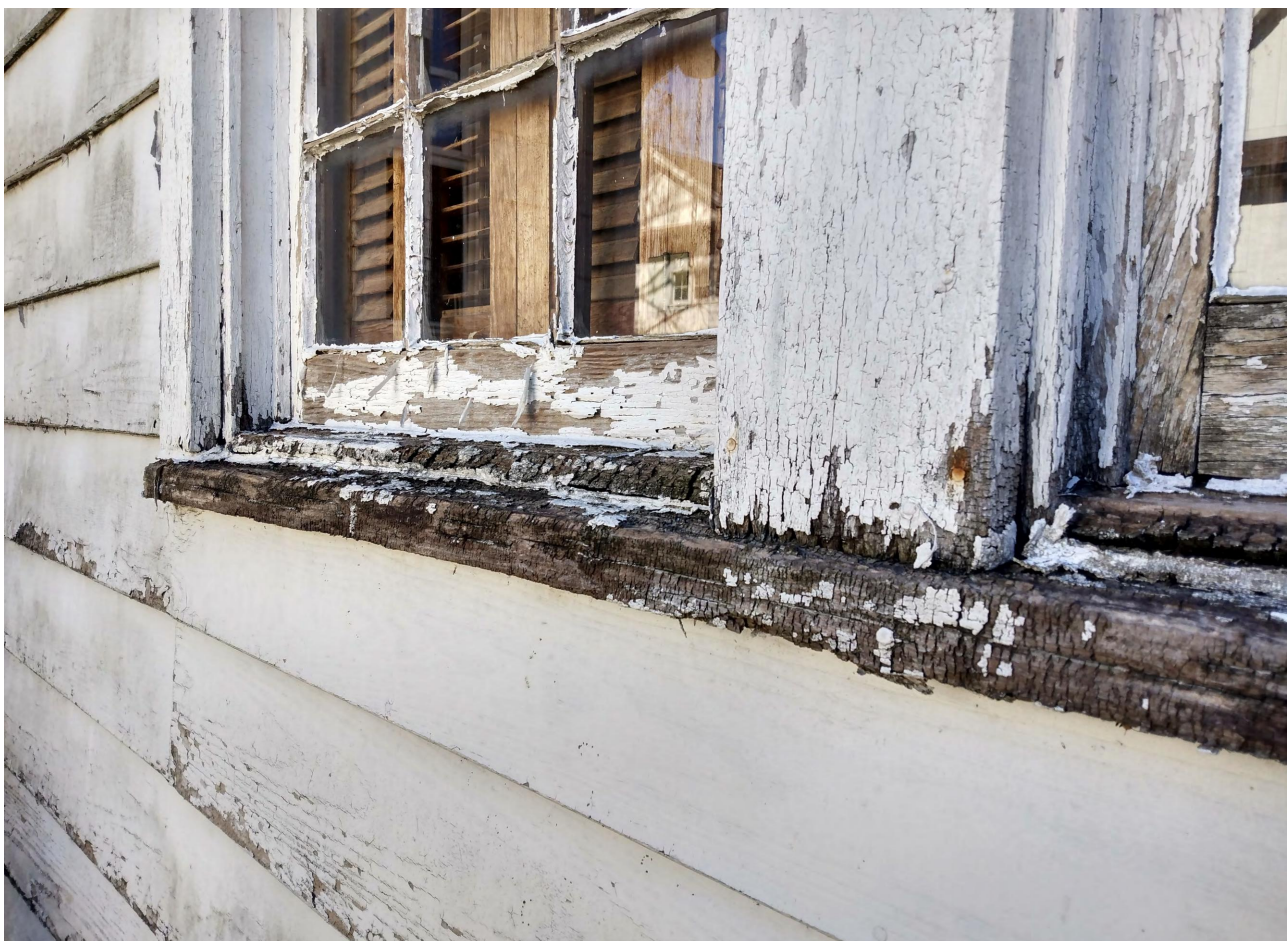
DETERIORATED WINDOW & SILLS
