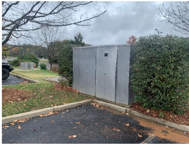
Existing utility water backflow system along subject front parking curb alignment (Looking Northwest towards Carothers from proposed building)
