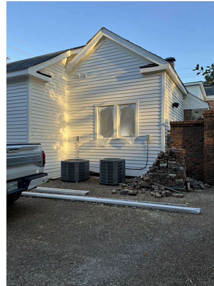
EXISTING REAR EQUIPMENT
