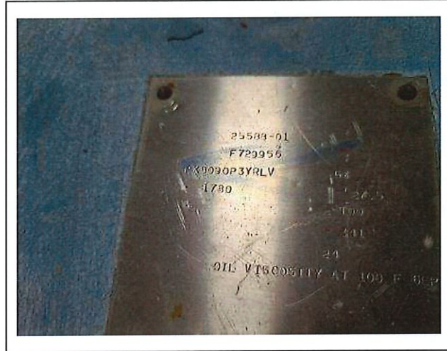
Picture #2: Unit Nameplate
